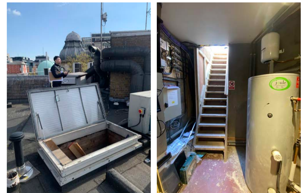
Current plant room with ladder access to roof level
