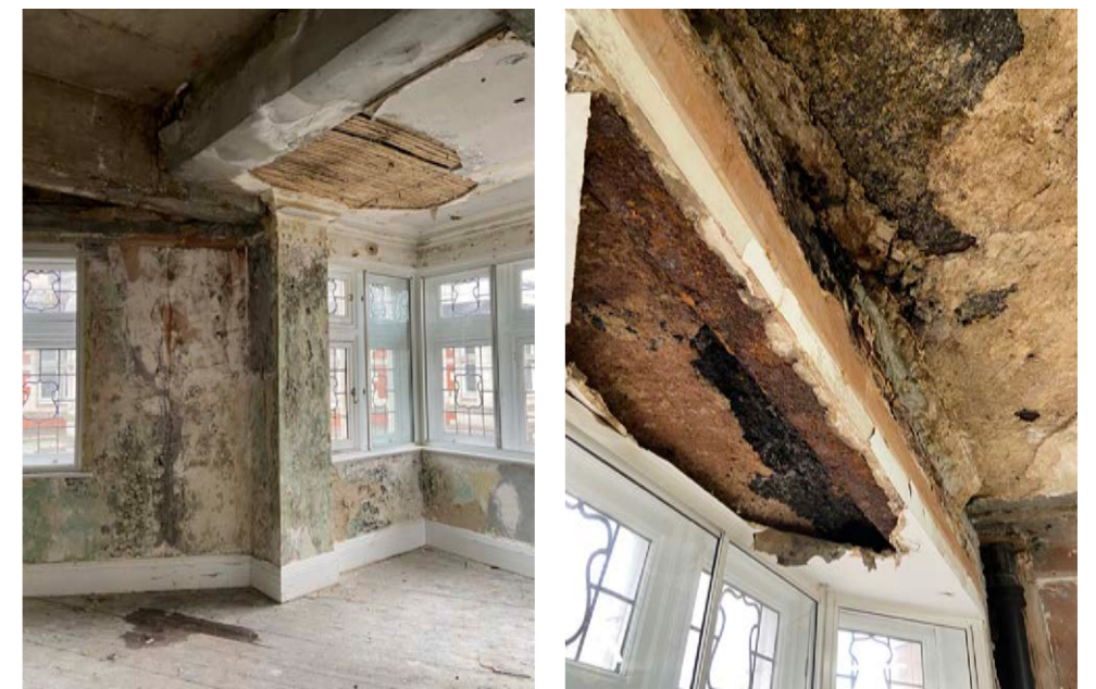
Evidence of water ingress within some window bays
