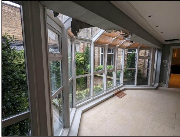
Figure 4.4: Ground floor extension, added in the 1990s, with conservatory style PVC framed windows
