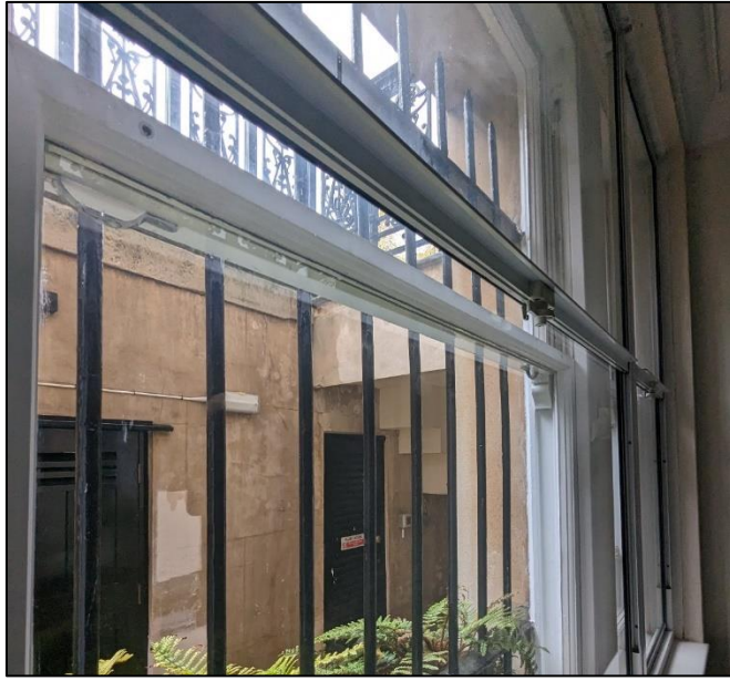
Figure 4.8: Secondary glazing with poor visual quality in the basement level front room
