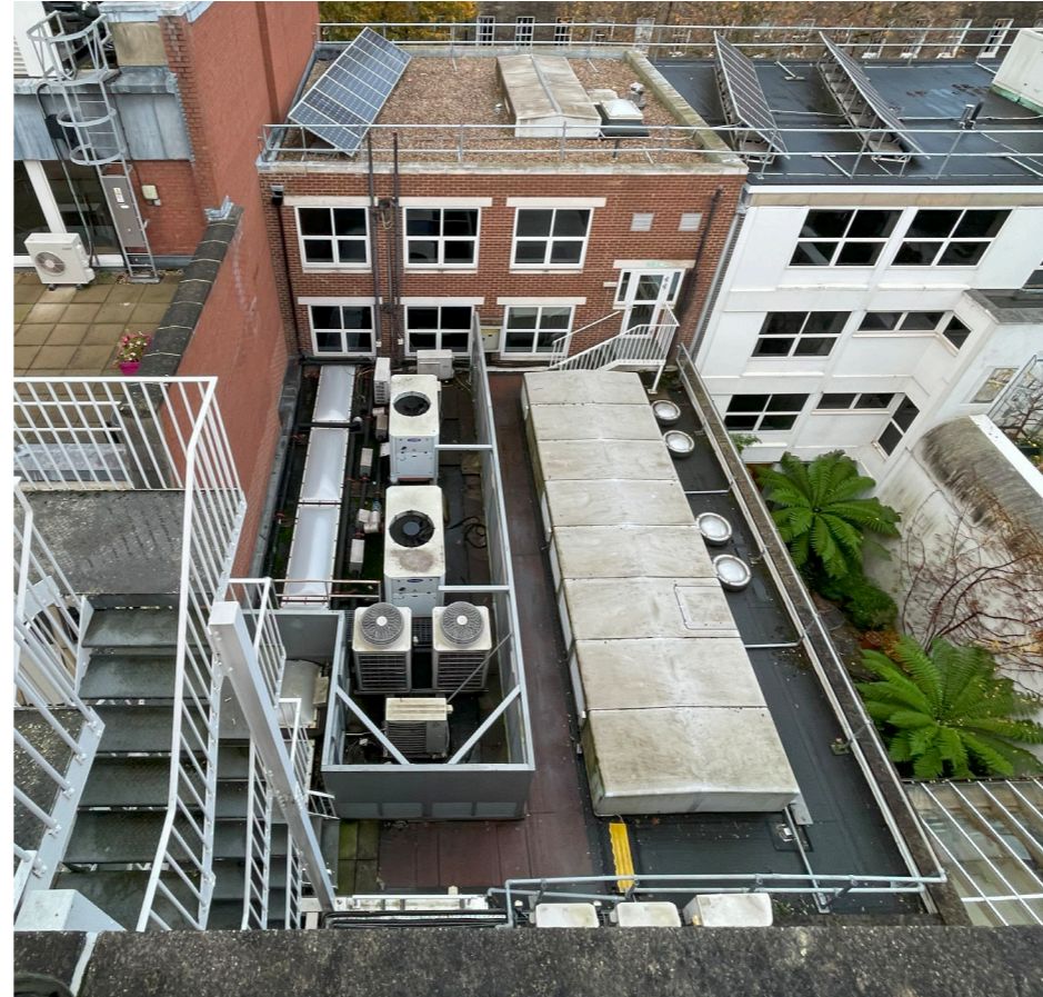
Plant equipment on 'link' structure roof
