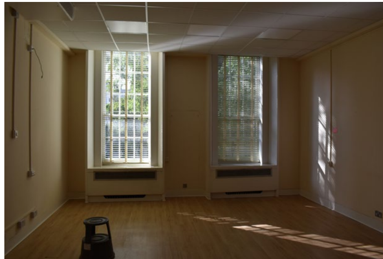
3.14 14 Bedford Row, first floor front room showing suspended ceiling cutting across top of traditionally-styled windows
