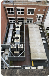
Existing plant level
