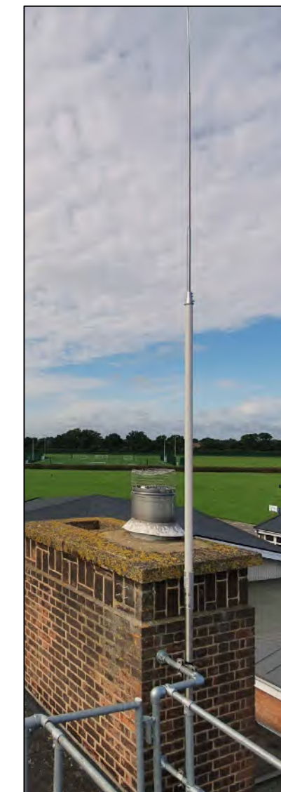
Example of HVI Mast
