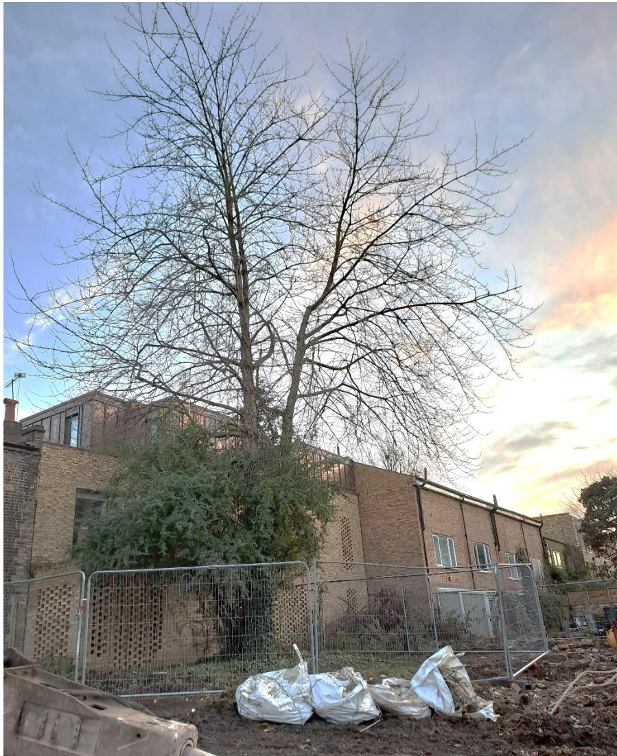
Photo 2 of tree protection fencing for T5. In correct location. Requires bracing with scaffold poles or diagonal struts.
