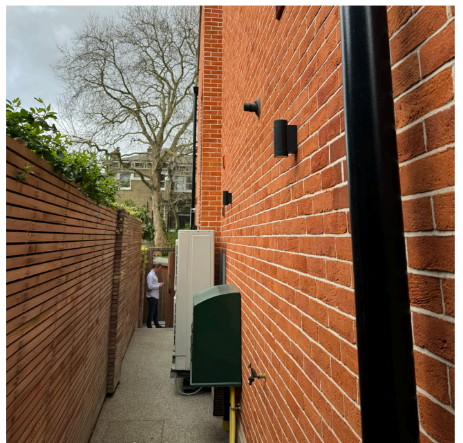
3. View of the condenser from the garden
