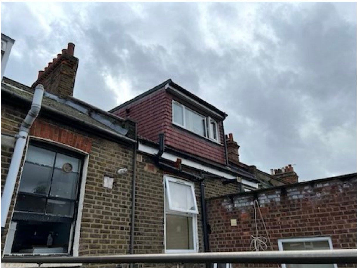
The above photo shows the adjacent rear dormer window, one of many in the terrace. To note in regards of the rear dormer windows is that they must be set in from the party walls.
