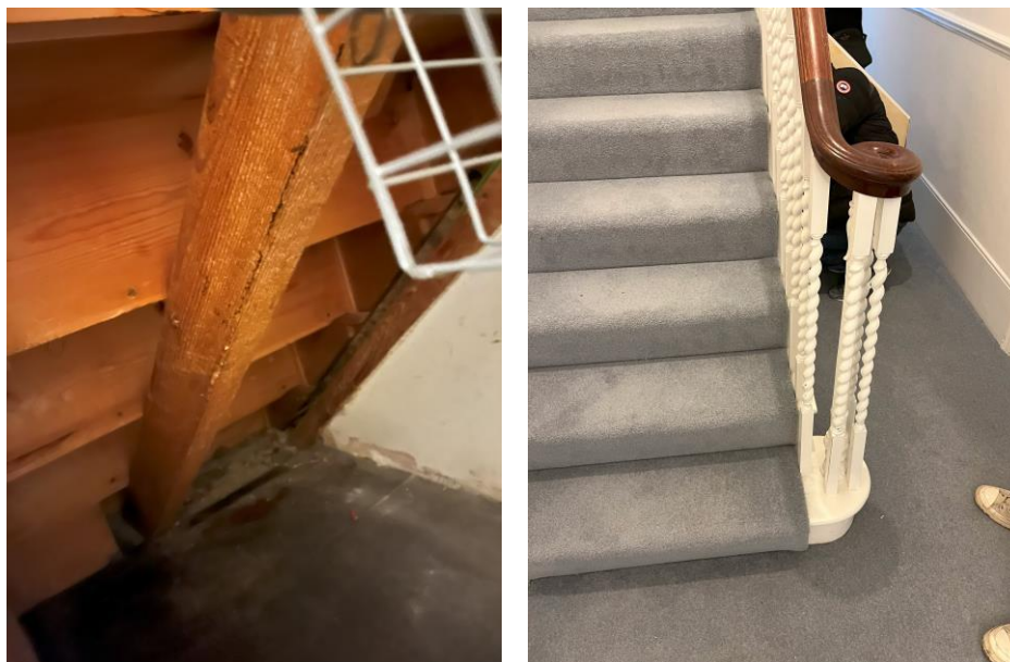
Figures 12 and 13: Existing staircase showing modern balusters (left) and modern construction (right)
