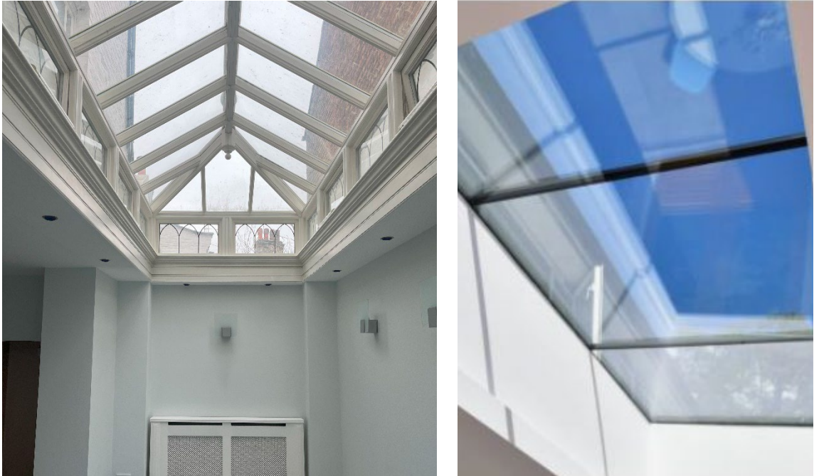
Figure 3: Images of Ground floor Roof light (left) and Proposed Replacement Roof light (right)
