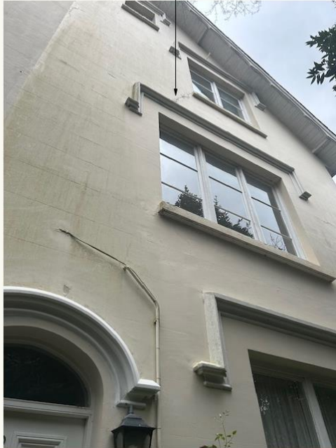
Cracks in the stucco finish on front elevation
