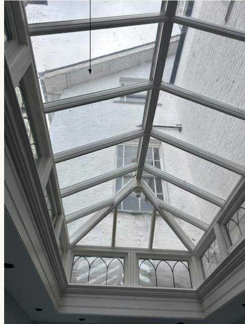
De-laminated non-original fascia to be replaced to match the original feature
