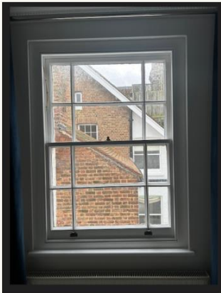
Non original frame, non original glass sash cord broken & rotten frames
