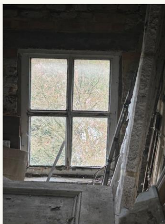
Original frame, non original glass window fixed shut
