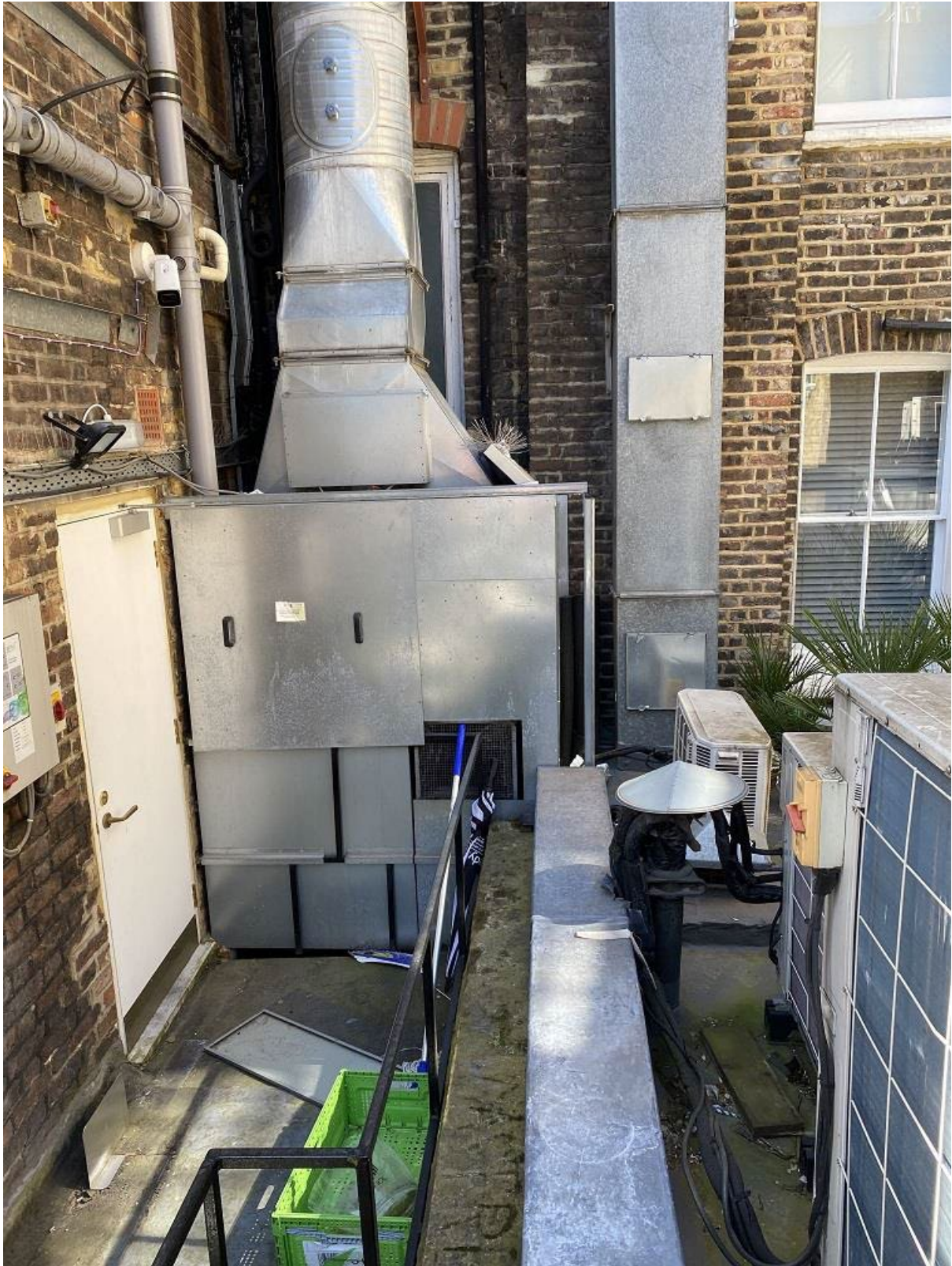
Photograph 5 –Plant at rear 10 Charlotte Street.
