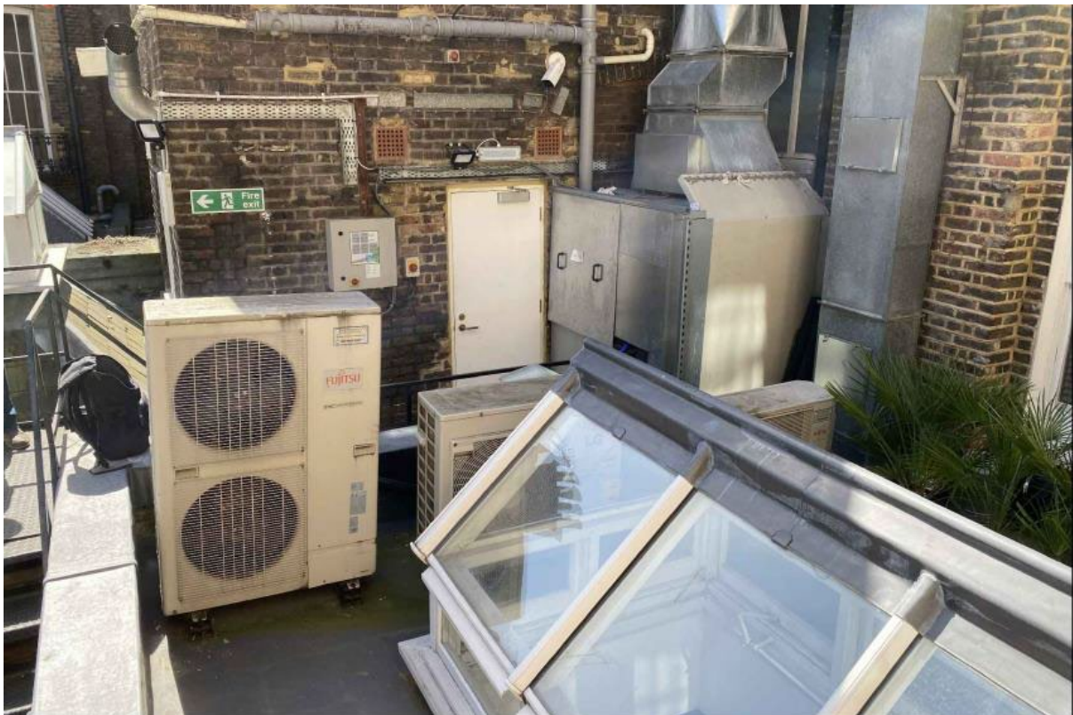
Photograph 4 – Rear of 10 Charlotte Street looking towards 8 Charlotte Street showing the existing roof plant.
