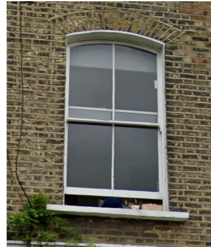
White Painted timber sash windows with white plaster detailing to sill. Soldier course brickwork lintel
