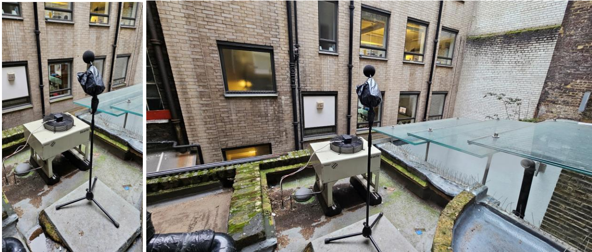
Picture 2: external cellar cooling unit - noise measurement position
