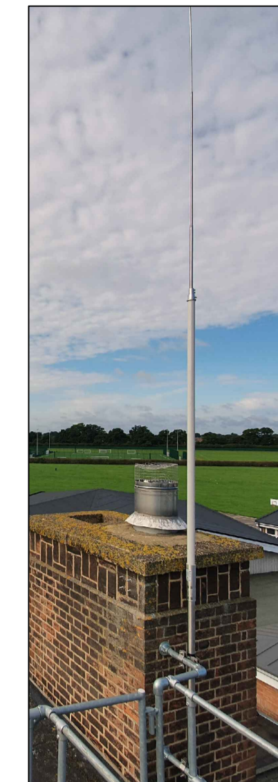
Example of HVI Mast
