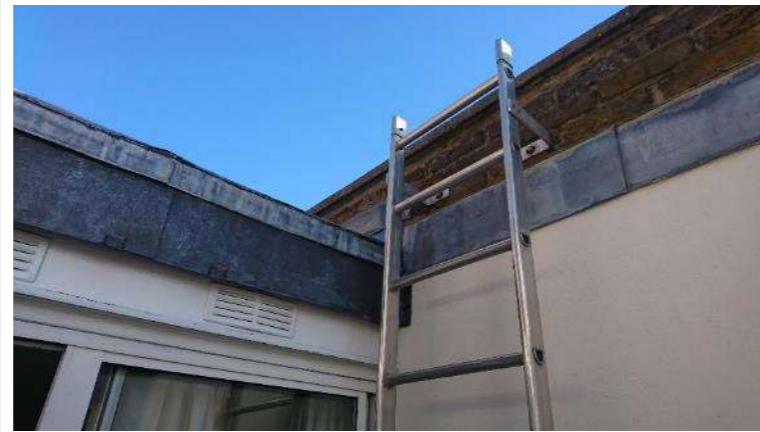
Photograph 49: No 159 party wall
