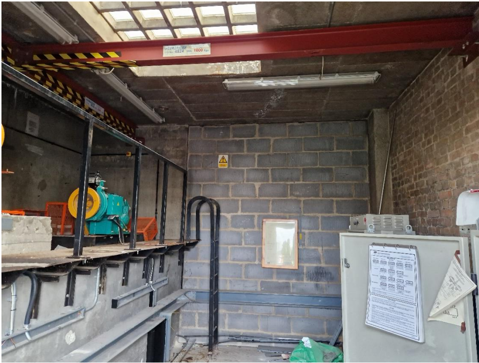
Photograph 3: Internal area of plant room on the roof of building B1
