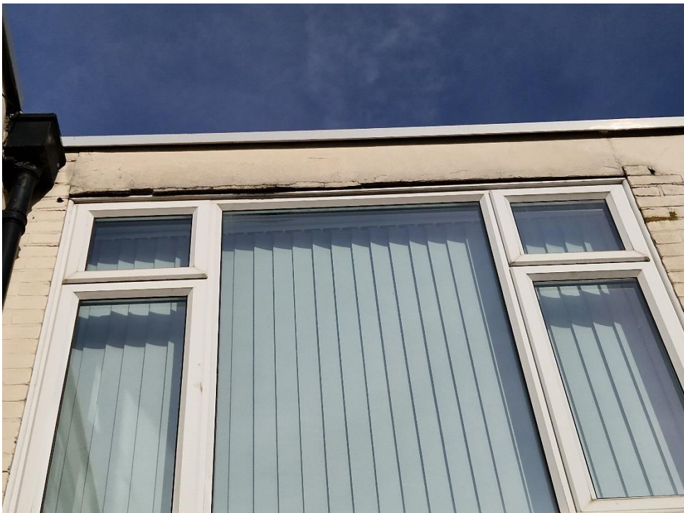
Photograph 6: Damage above window of the brick-built office-extension
