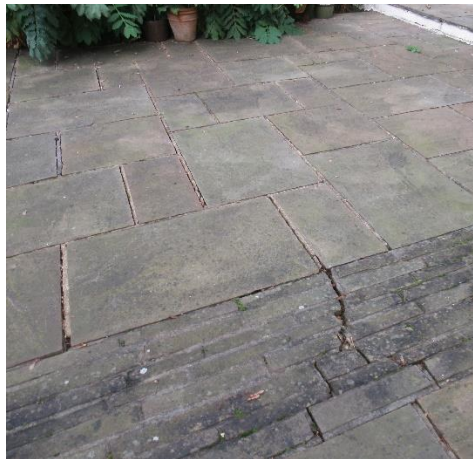
Figure 6: Cracking and damage to paving in need of repair and replacement.
