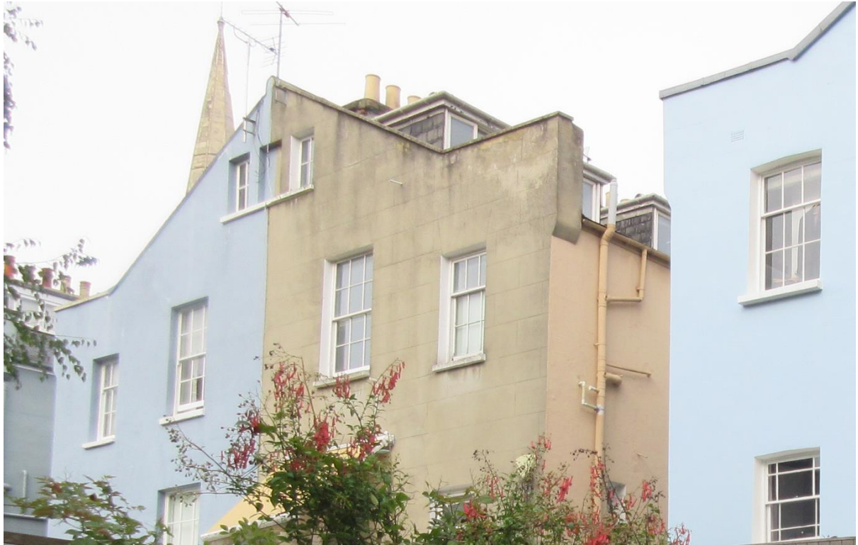
Figure 3: The rear elevation of 9 Provost Road in December 2023, showing its as-built state. The house takes the same form as 3 Eton Villas, is in the next street, and is by the same architect, but is five years older.
