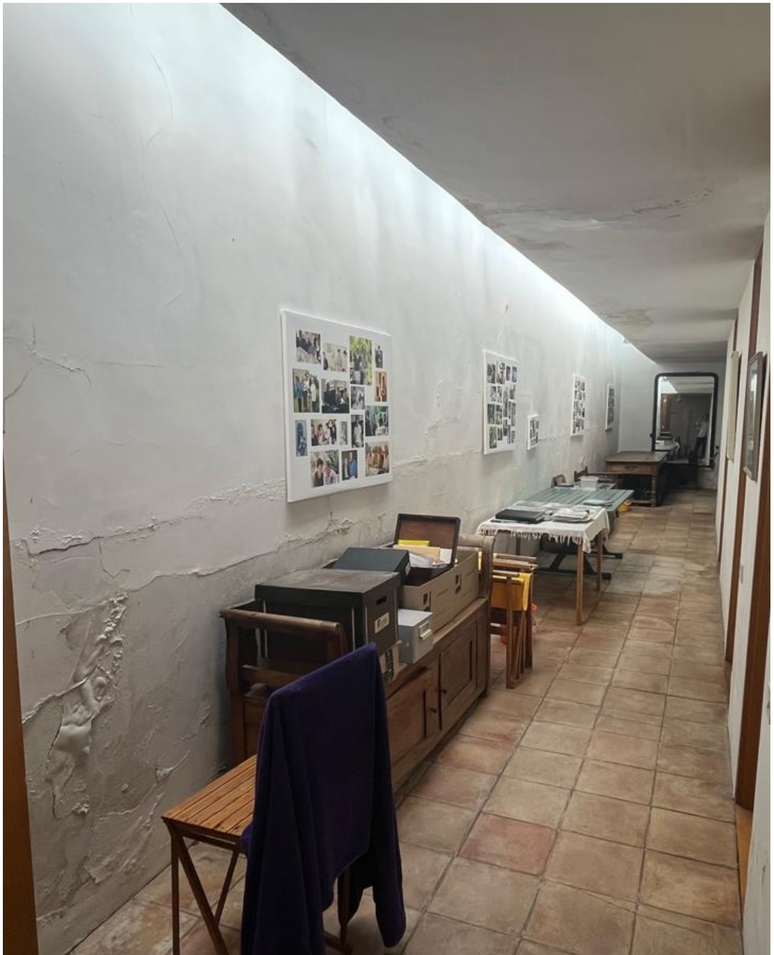
Photo showing cracking to perimeter wall
