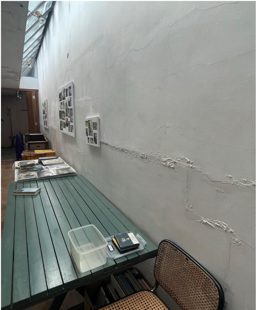
Photo showing cracking to perimeter wall
