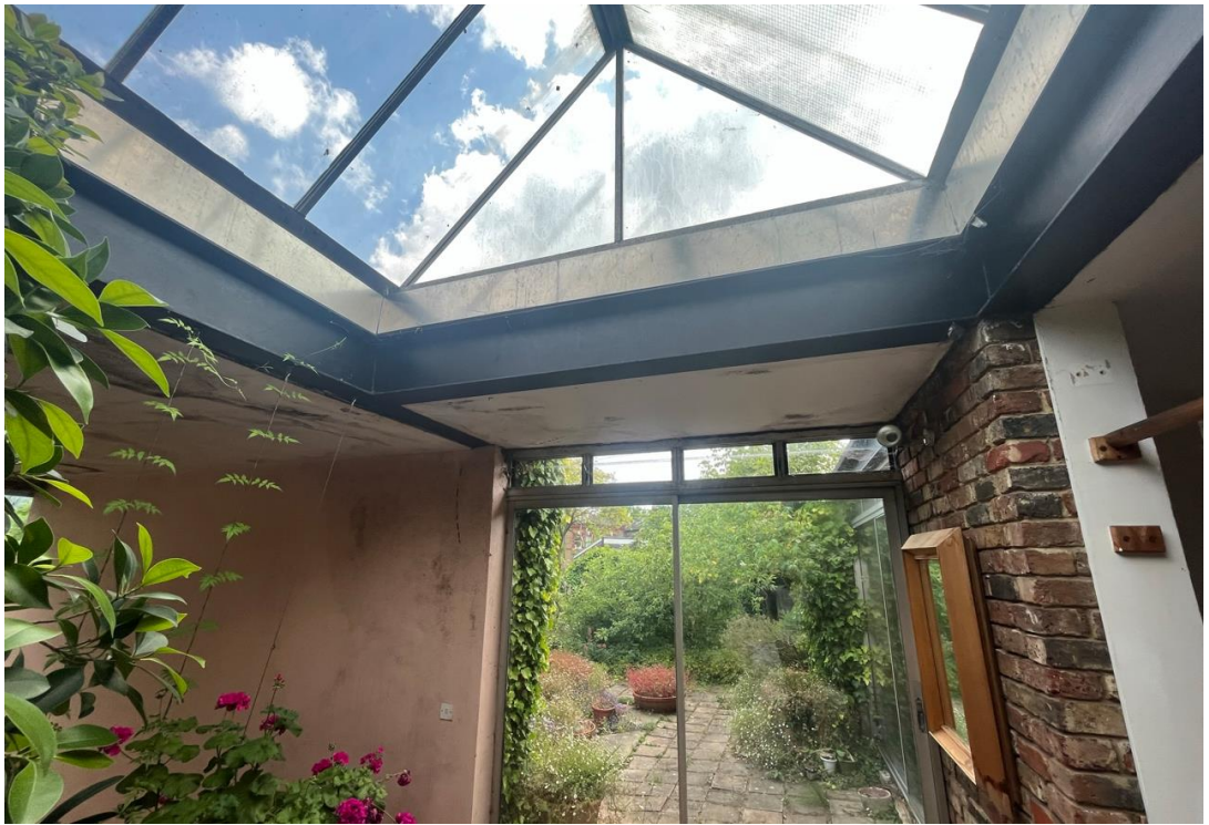
Photo showing poor condition of roof and walls
