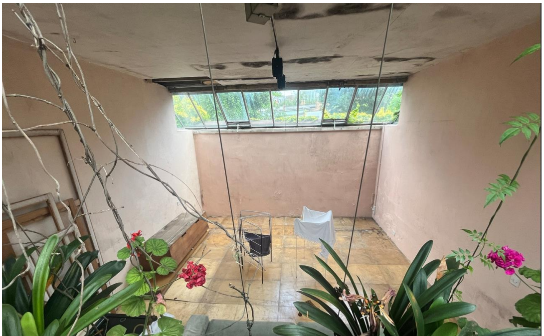
Photo showing poor condition of roof
