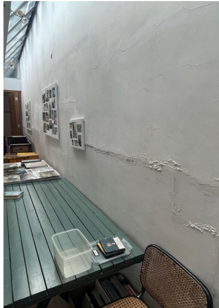
Missing and/or failed DPC/DPM to all main external walls.
