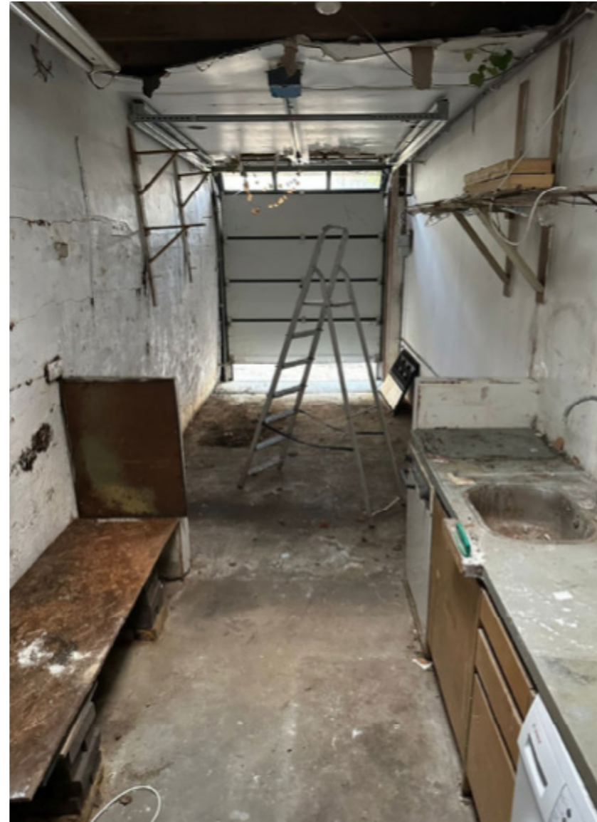
Roof to garage in very poor condition with leaks due to roofing system failure.
