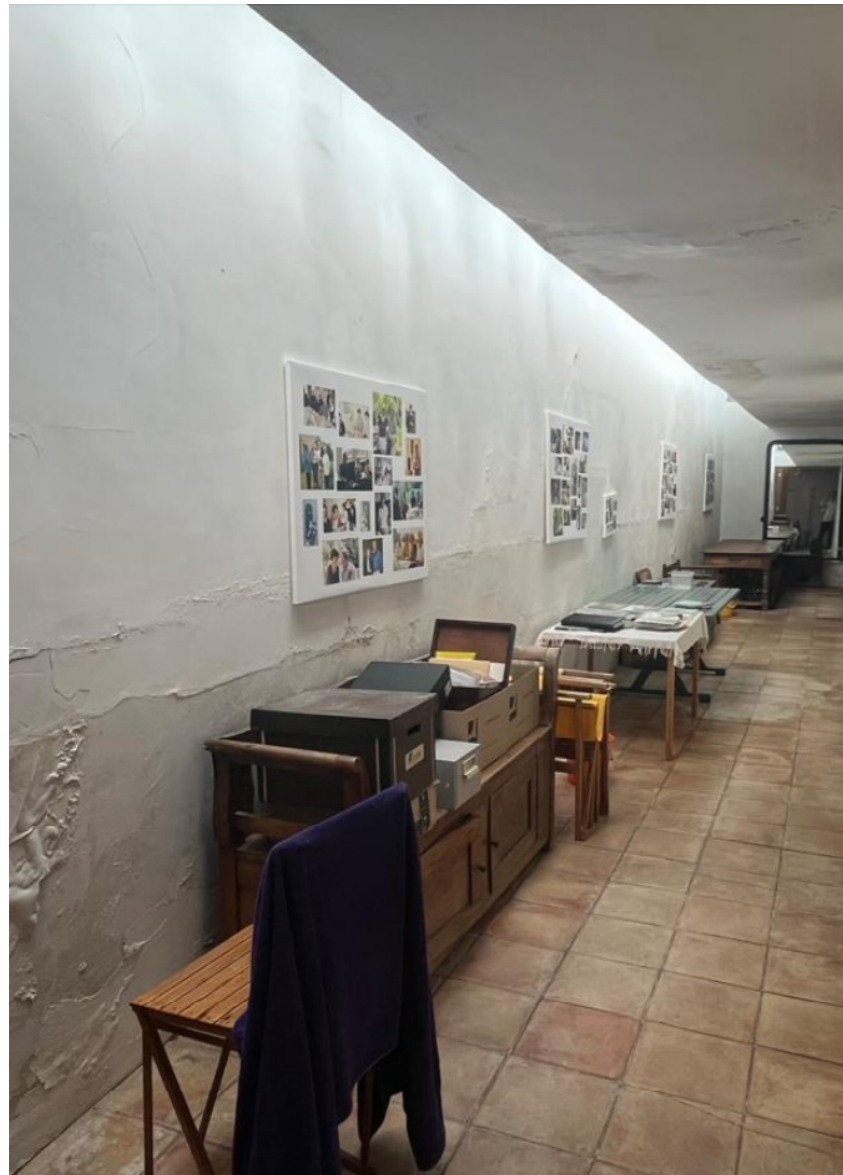
Corridor with main party wall with neighbouring site in very poor condition with signs of large cracks.
