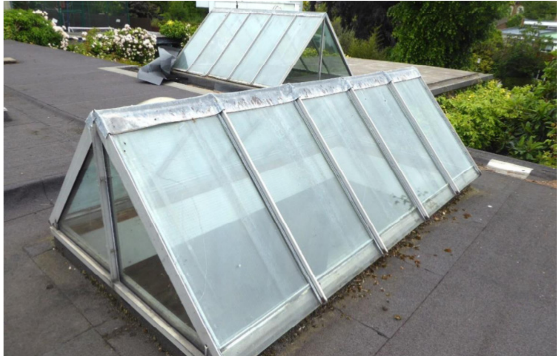
Glazing to rooflights showing signs of cracks and failure to system with evidence of poor maintenance/repairs.
