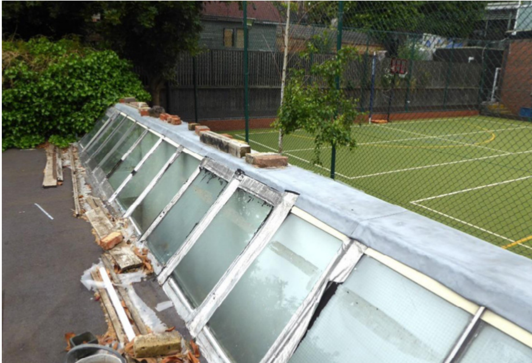
Area of rooflights along corridor in very poor condition with need to replace entirely (see Planning History).
