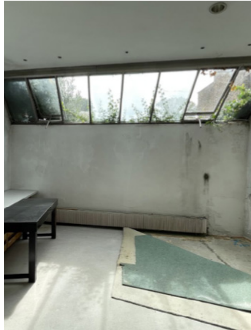
Failure of glazing systems throughout, including evidence of vegetation growing through window framing.
