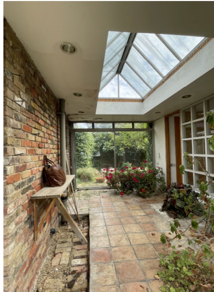
Tiling missing and signs of issues with underfloor heating services.
