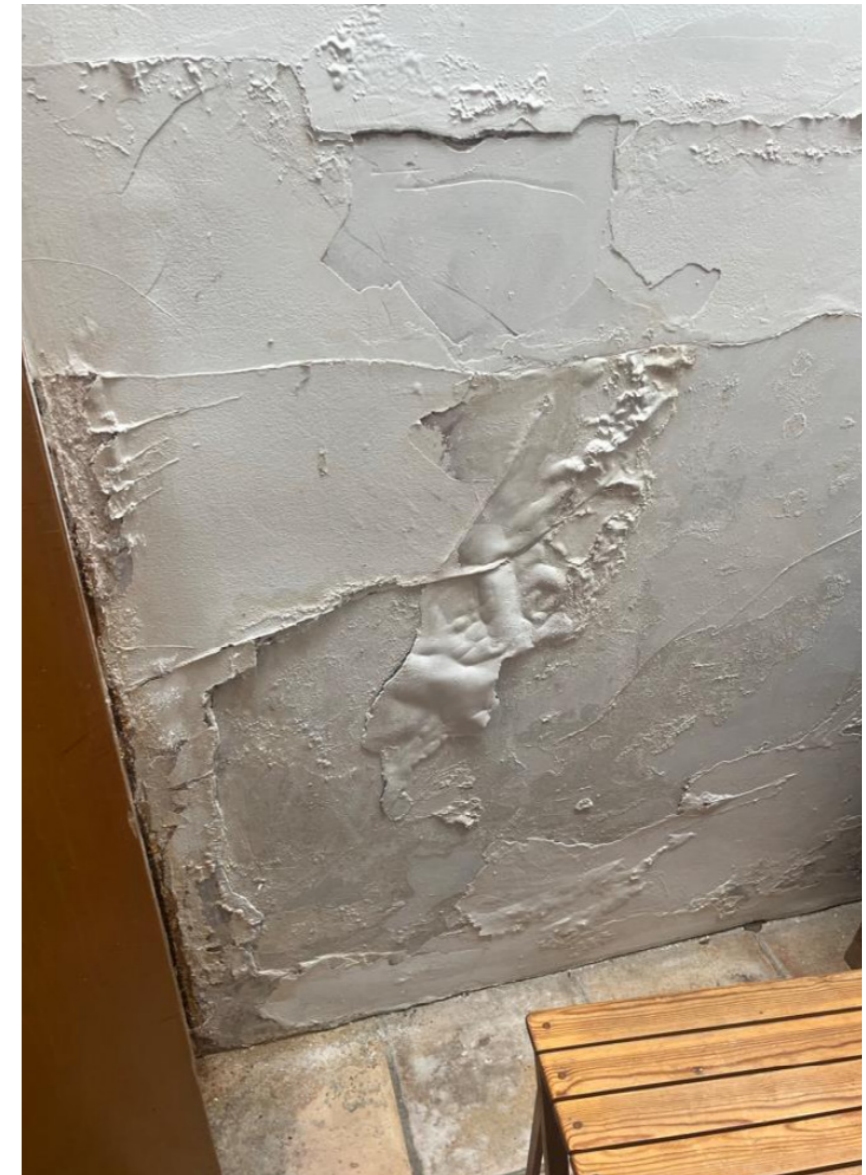
Issues with damp on all external walls and some interior rooms.
