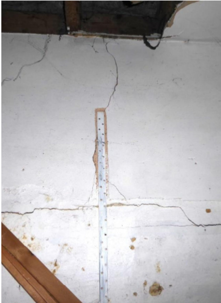
Garage construction poor with major walls showing cracks.
