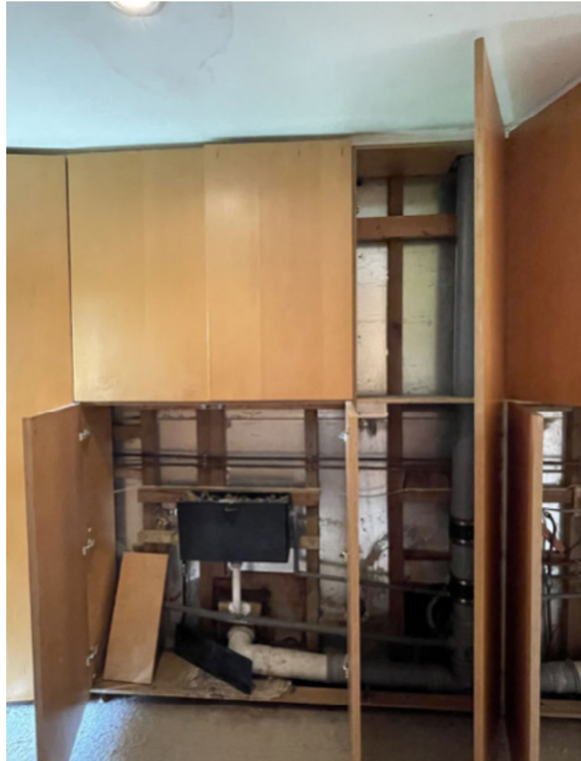
Waste from bathrooms in poor condition with unconventional location for noisy cistern in adjacent bedroom.
