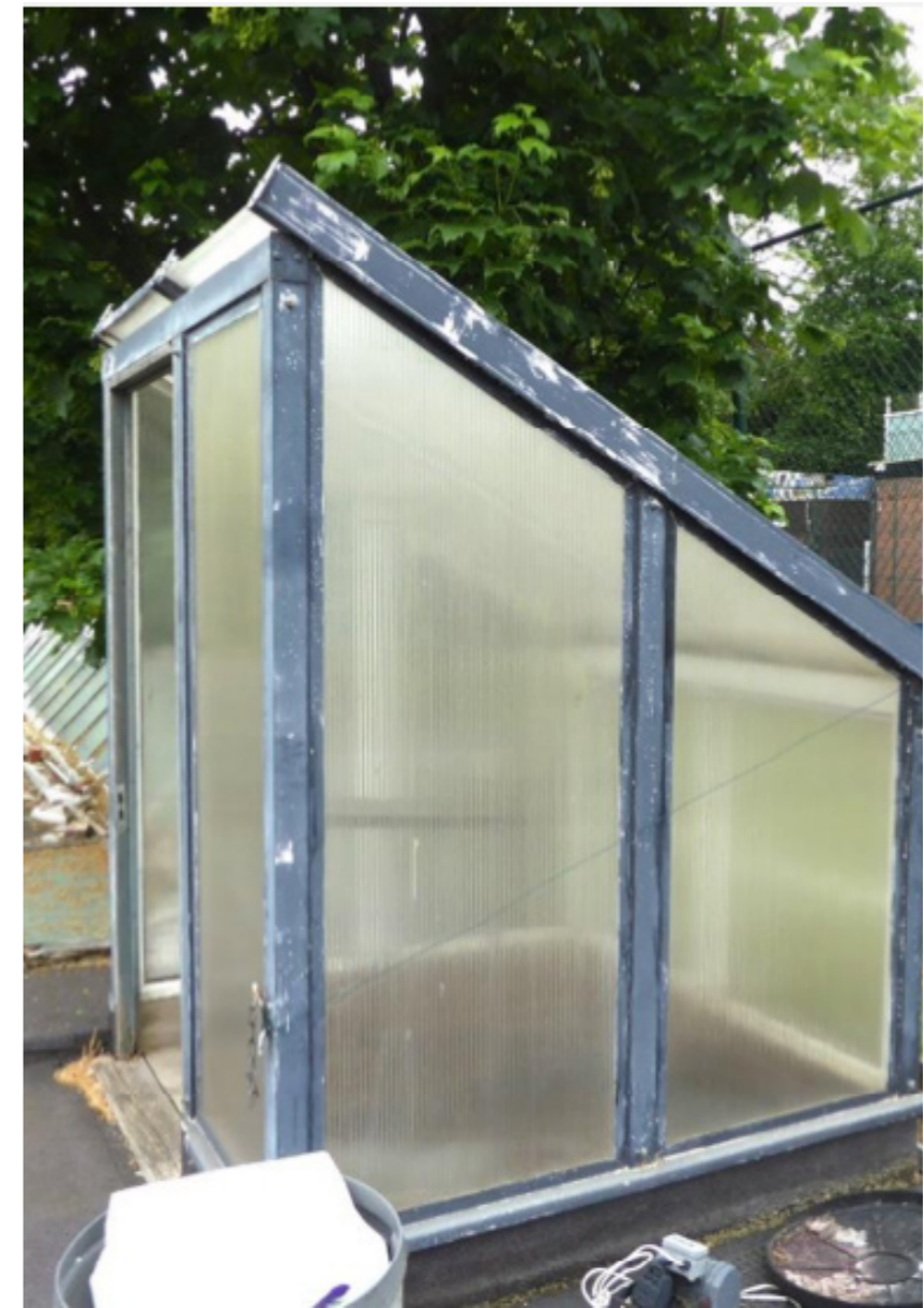
Roof access and structure to stair in poor condition.
