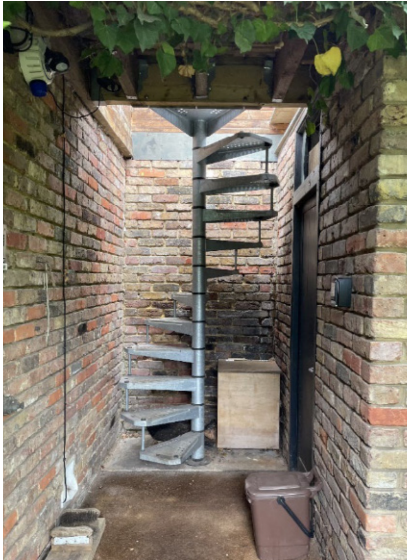
Access to roof from stair currently unsafe due to no handrail.
