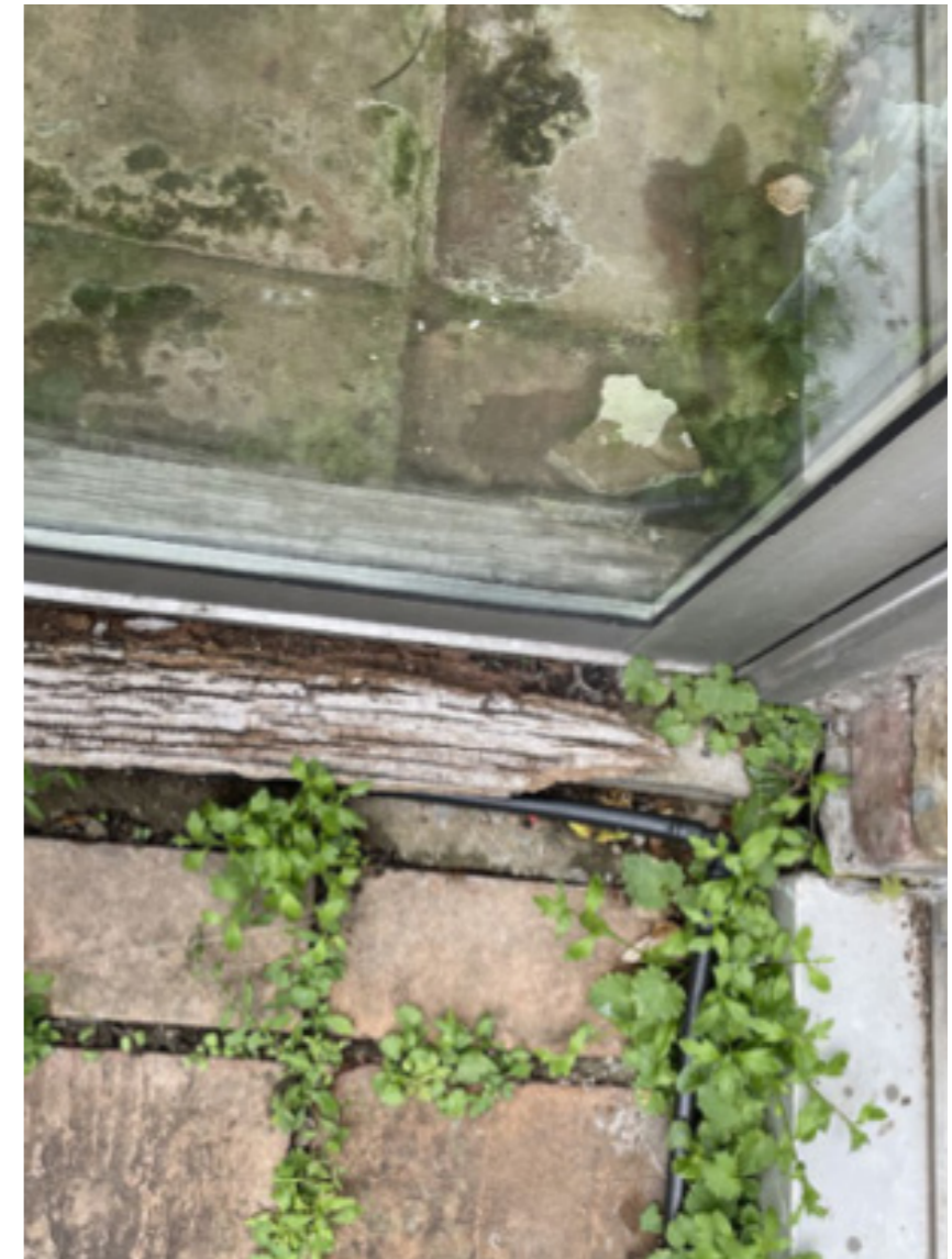
Sliding glazing doors and windows currently jammed due to movement and failed systems.
