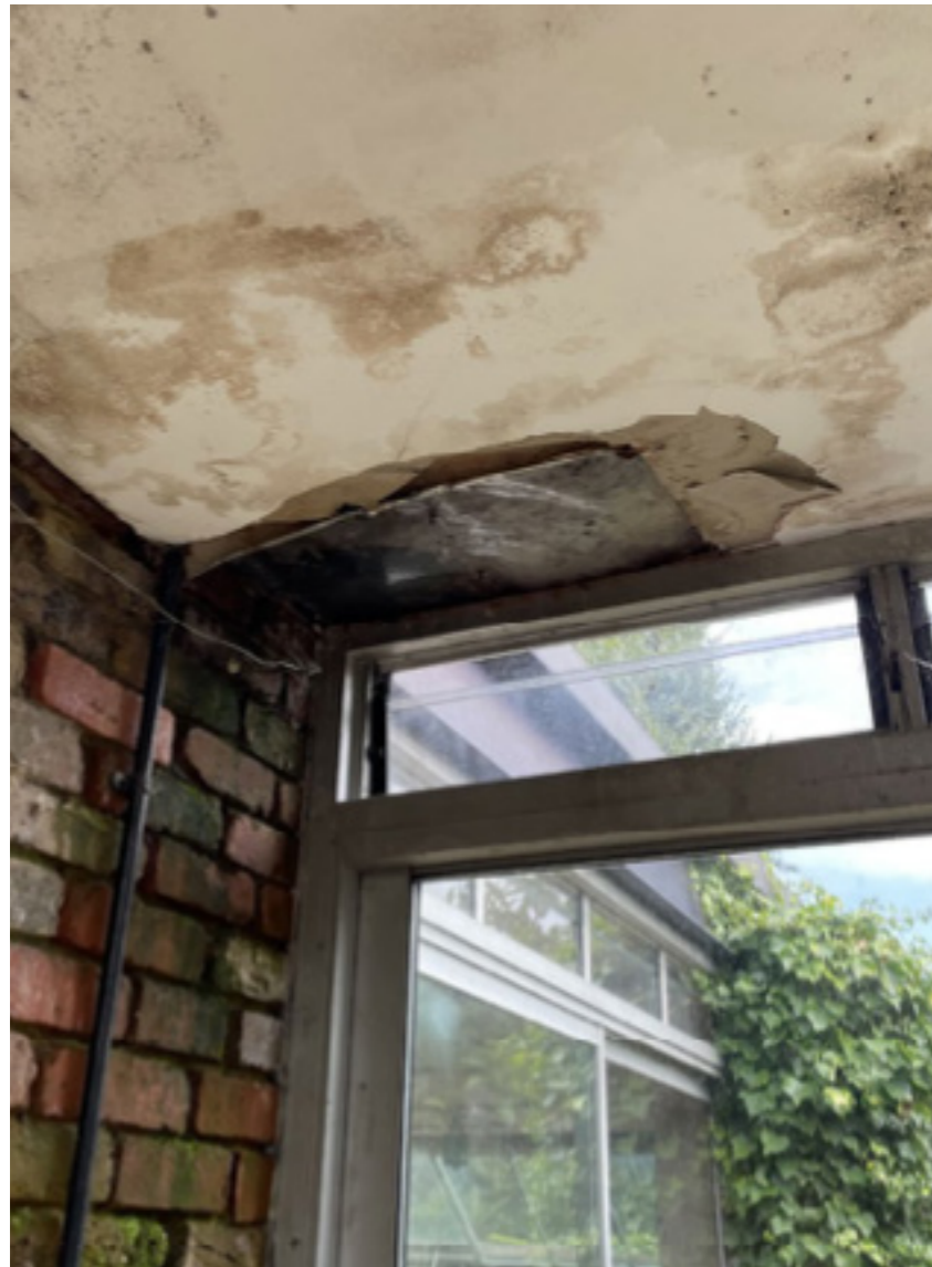
Issues with leaks from existing roof and connections with walls where they meet outside.
