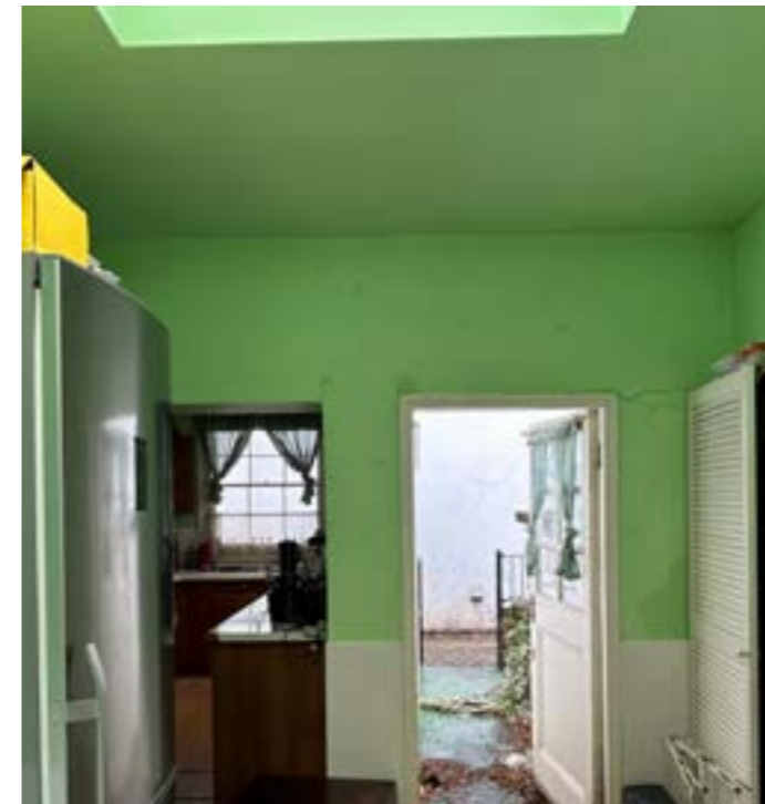
Figure 4.10 The ground floor pre-listing extension rear wall also showing signs of structural failure and dampness (see crack along the door lintel).
