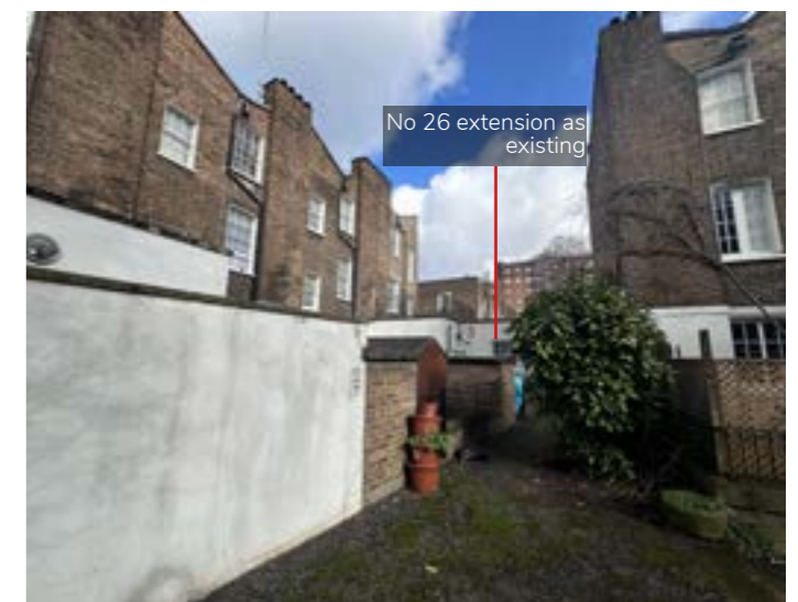
Figure 4.6 Rear view of the extension to No 26 taken from the communal garden.
