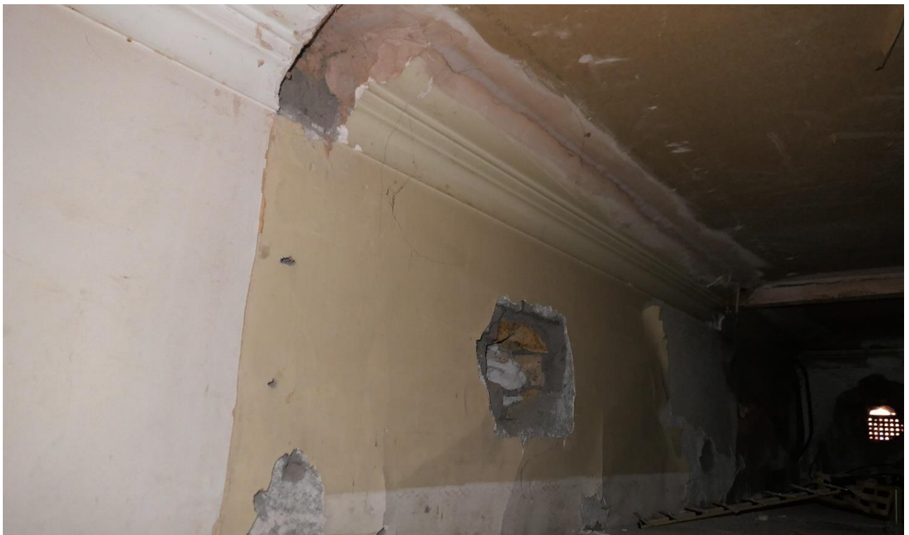
Photo 1: The suspended ceiling, with what appears to be the residual original cornice, in the former large front ground floor room of 33 Ferncroft Avenue.
