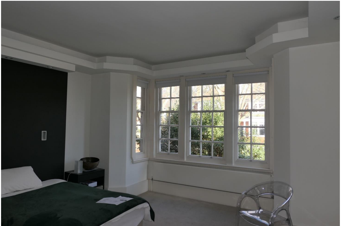
Photo 9: The very odd and heavy-looking, projecting 'cornice' at the front room of the first floor flat.
