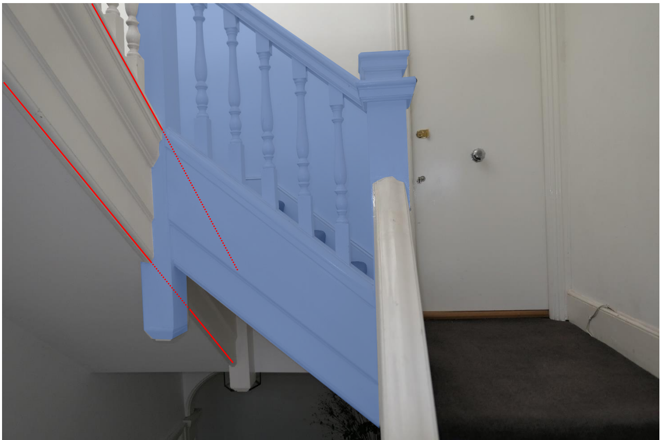
Photo 7: A photo of the staircase from the ground floor landing, with the original flight highlighted in red, and the inserted flight highlighted blue.
