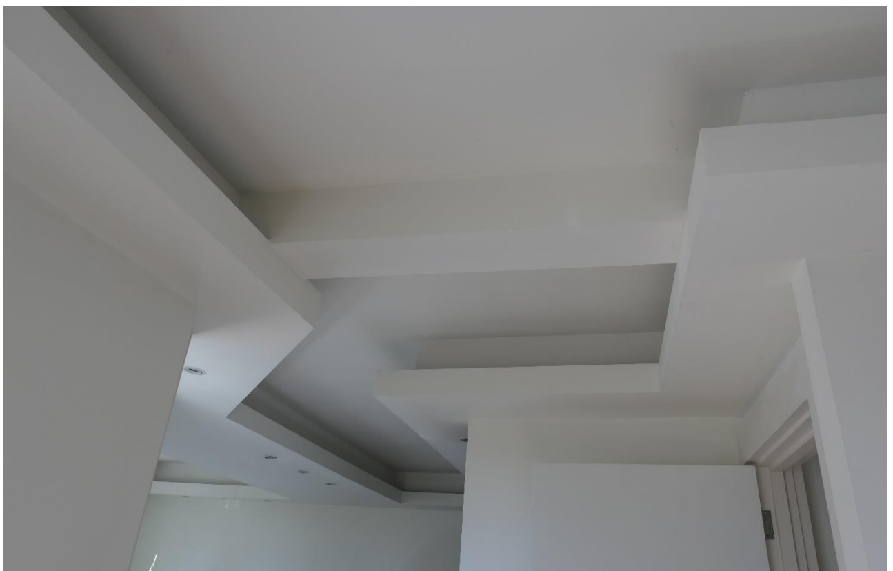
Photo 10: The very odd and heavy-looking, projecting 'cornice' at the rear of the first floor flat.
