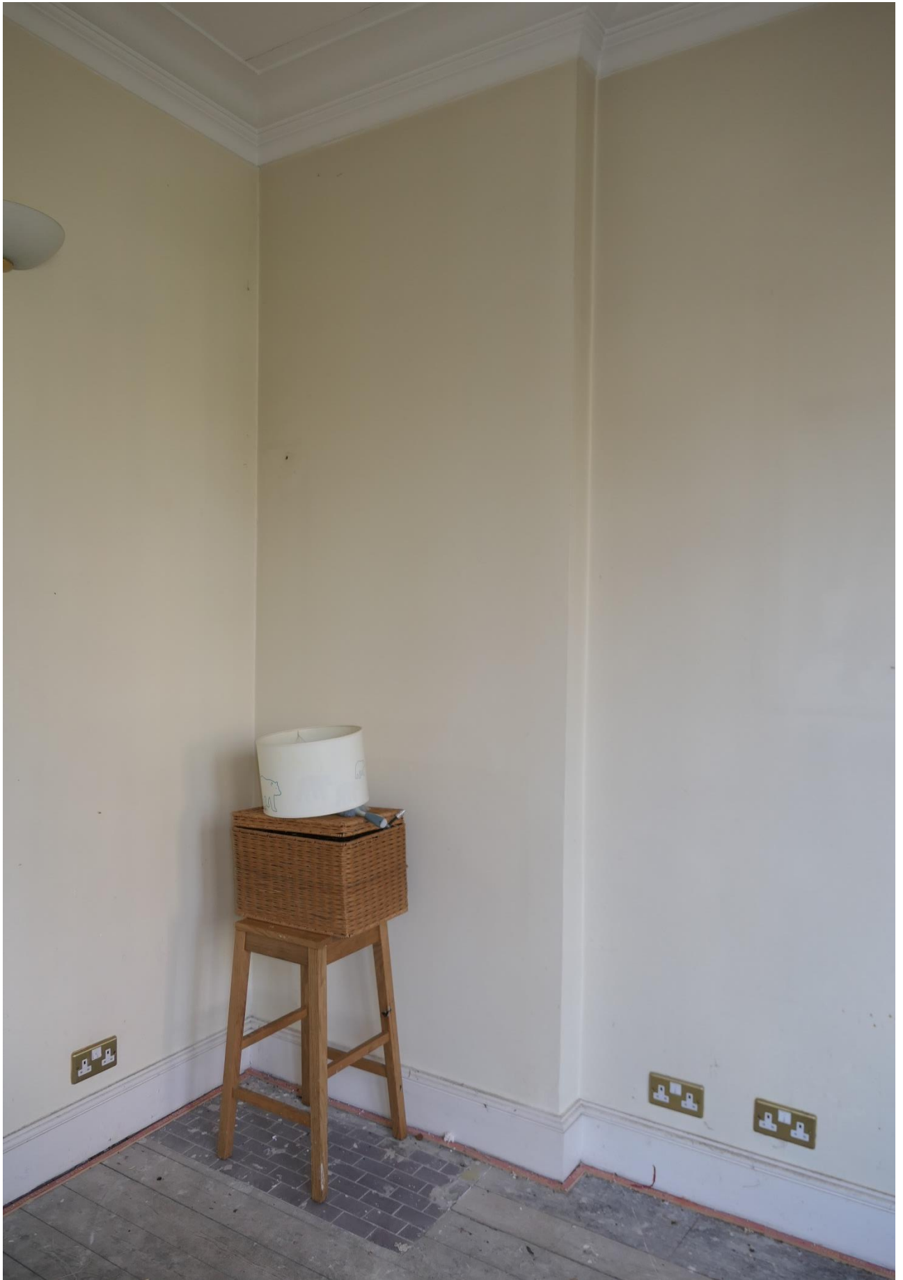
Photo 2: The chimneybreast in the former large front ground floor room of 33 Ferncroft Avenue is overlapped by a partition; the (presumed original) tiled hearth can be seen on the floor.
