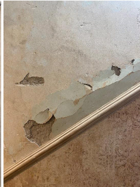
Loose and Damaged Plasterboard
