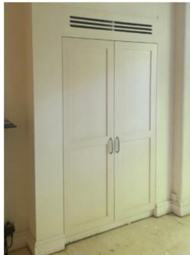
Lower ground floor non-original architraves and skirting to be replaced
