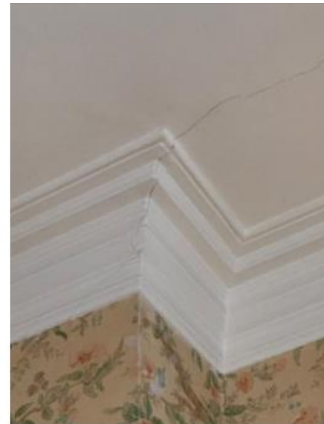
Non-original cornices and architraves on the ground floor to be replaced
