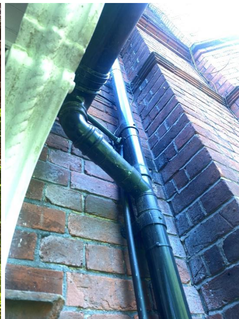
Non-Original Black UPVC Soil Vent Pipes
