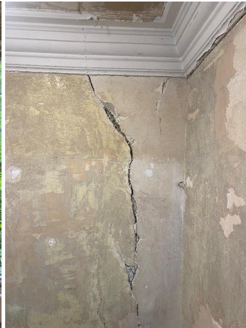
Prominent Cracks in Plasterboard
