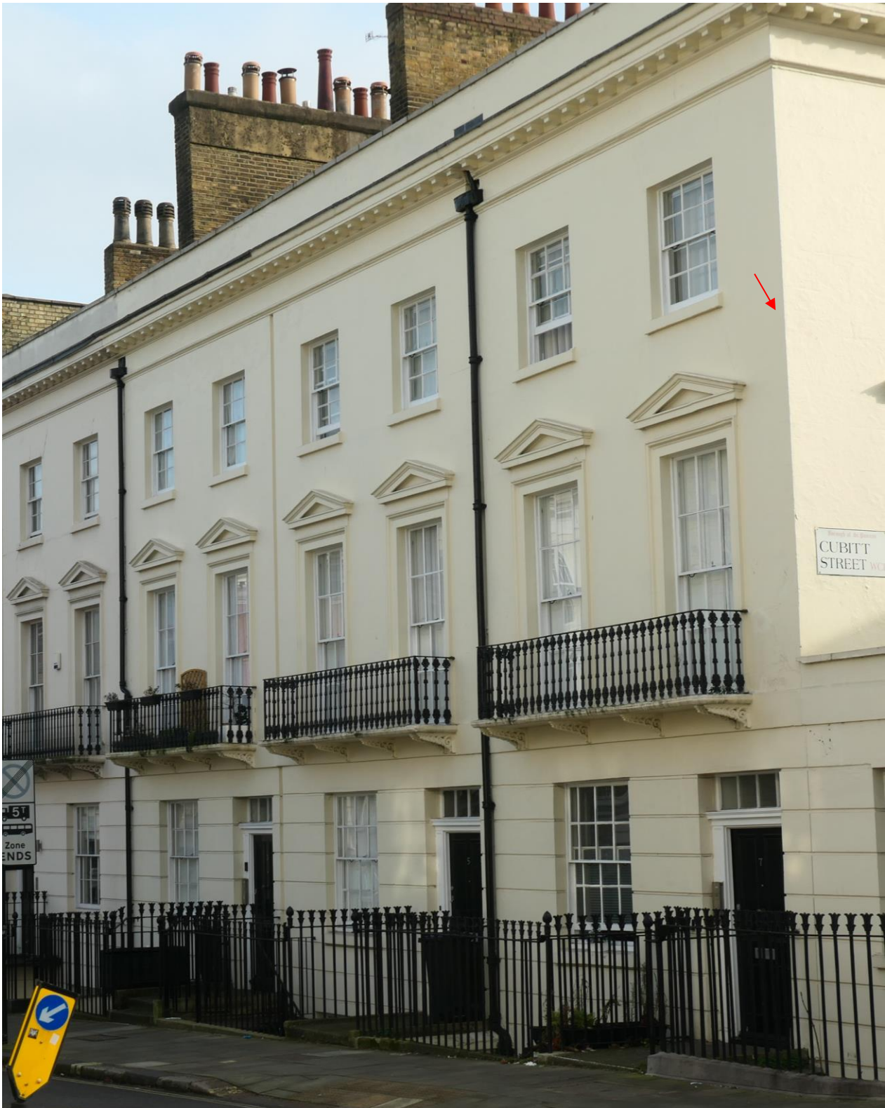
Photo 8: A detail of 1-7 Frederick Street, showing the absence of a vertical channel at the end house. The arrow shows where the channel would have had to be located, if there was one, and it can be seen how odd that would have looked.
