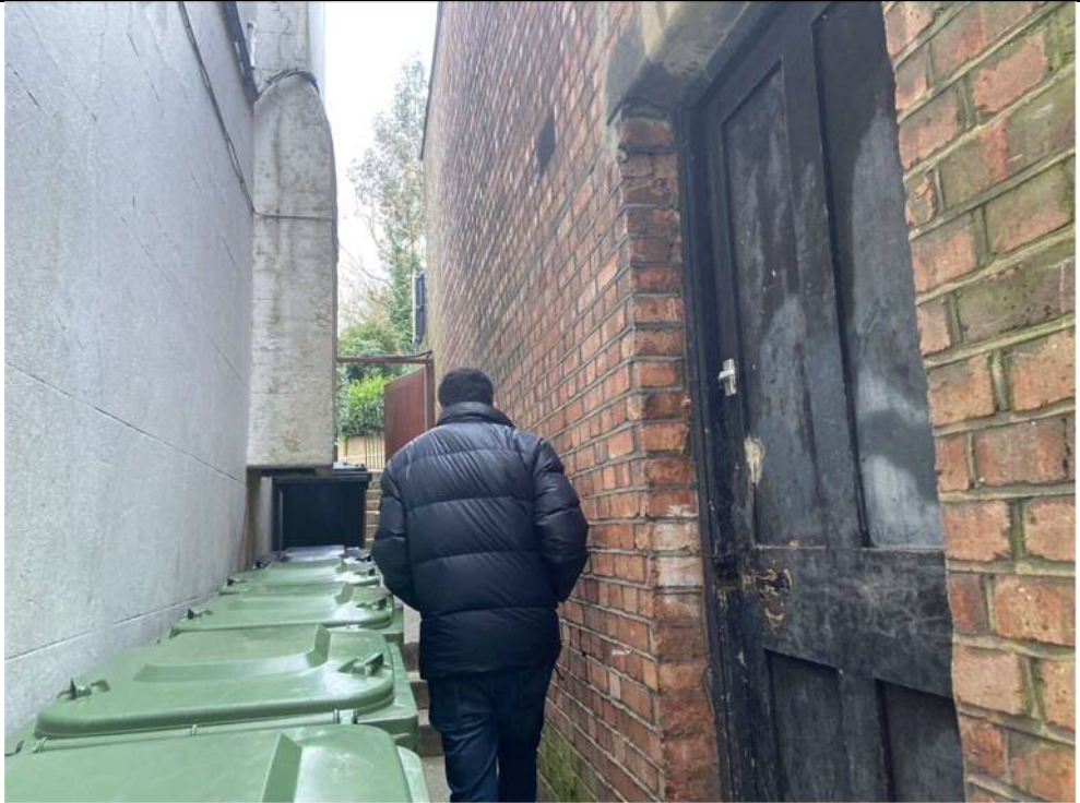
Photo 4: W boundary of site, photo facing N. Small alley way leading from the front of the garages to the rear. Small paved area with some vegetation.
