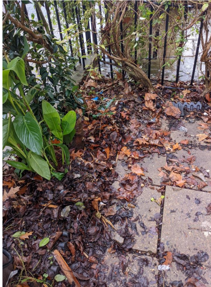
Concrete paving stones in disrepair and flowerbed
