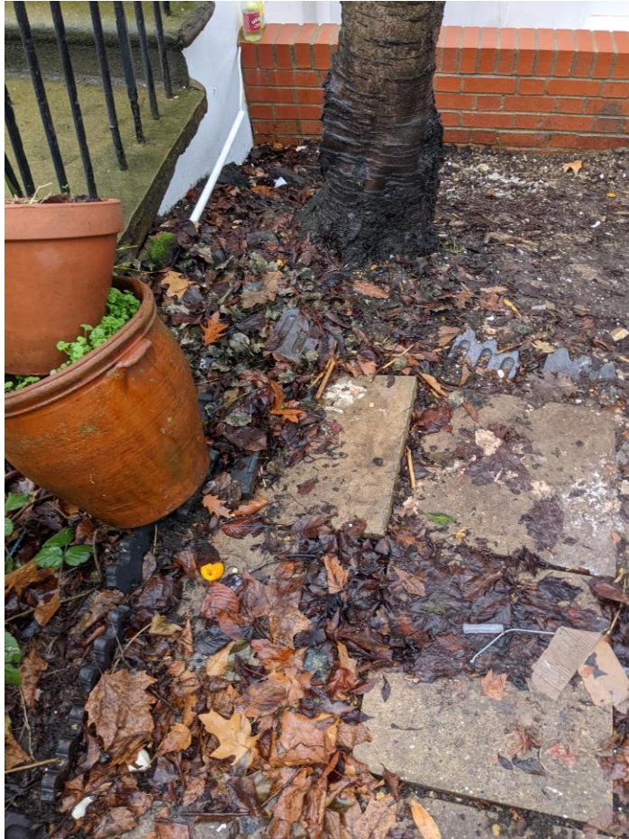
Concrete paving stones in disrepair
