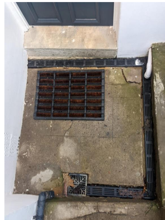
Existing footwell drain with linear drain surround
