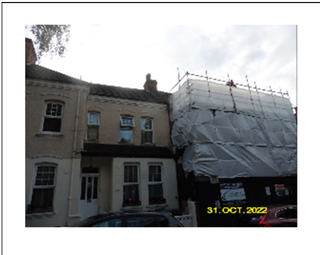
Front scaffold with No.165 seen on the left, note this scaffolding is fully sheeted and was restrained by a structure that had since been removed, leaving it inadequately restrained and dangerous.
