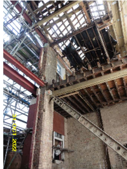
The remains of the front façade being restrained by a raking slimshore with shallow founding conditions, which would not permit the proposed excavation to take place.
