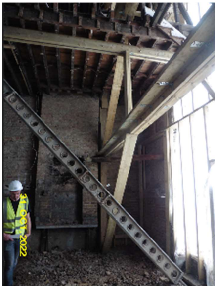
Unorthodox timber framing in place which was not founded at depth, which would allow for the proposed excavation to take place. Further raking RMD slimshores were not founded at depth
