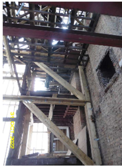
Unorthodox timber framing in place which was not founded at depth, which would allow for the proposed excavation to take place
