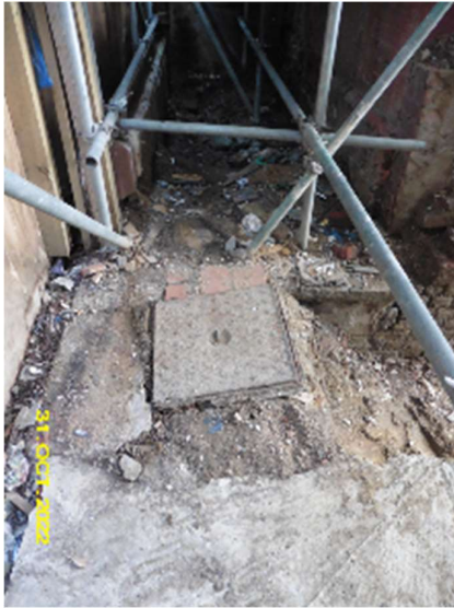
Scaffolding was found to lack baseplates and was placed on timber boards which had since begun to rot.
