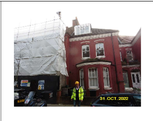
Front Scaffold with No. 161 on the right, note this scaffolding is fully sheeted and was restrained by a structure that had since been removed, leaving it inadequately restrained and dangerous.
