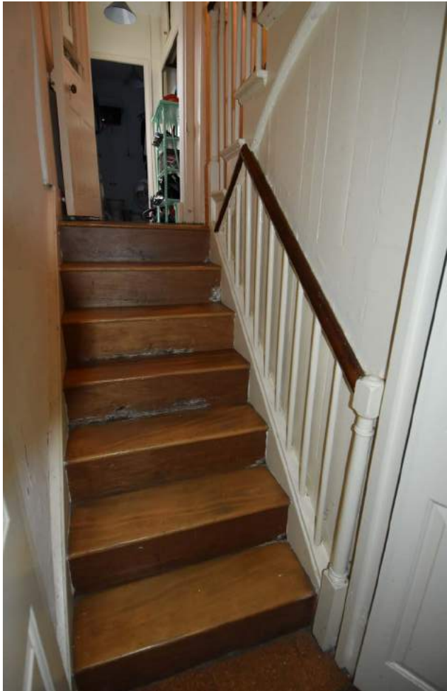
3.13 Staircase flight from lower ground floor to the half landing. The treads have been rebuilt (2023, Donald Insall)
