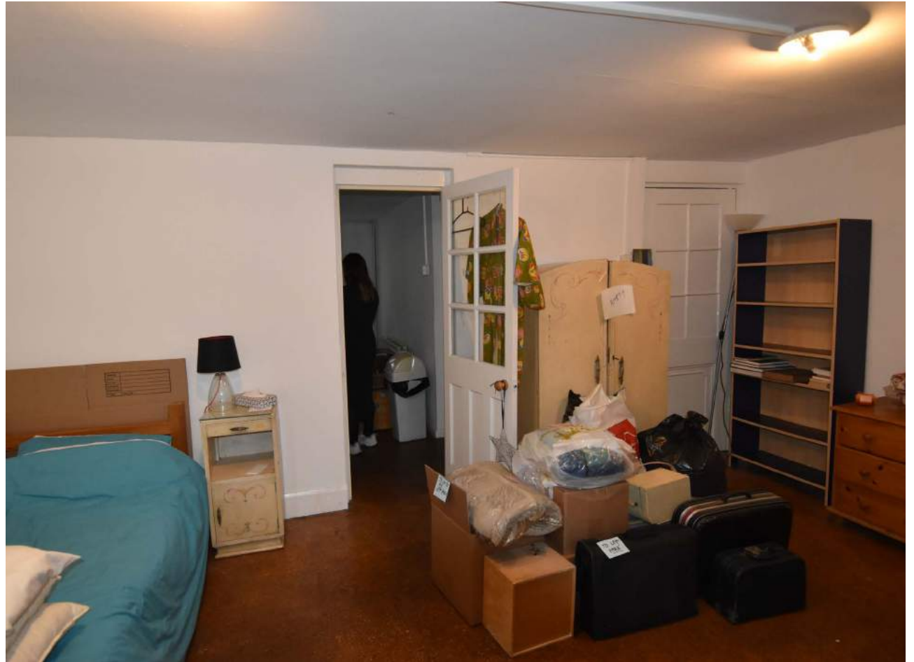
3.20 East wall in room LG3, showing the modern replacement doors (2023, Donald Insall)
