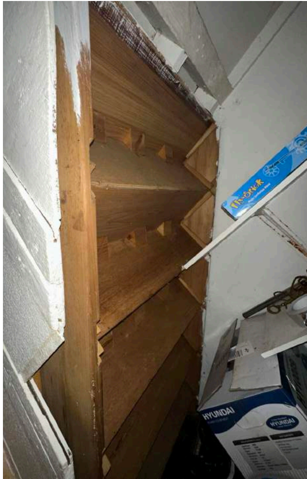
3.14 The underside of the lower ground floor stair in LG5, showing its modern construction (2023, Donald Insall)
