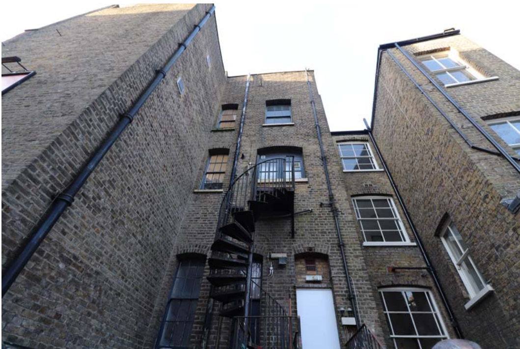
View of non compliant redundant spiral staircase.
