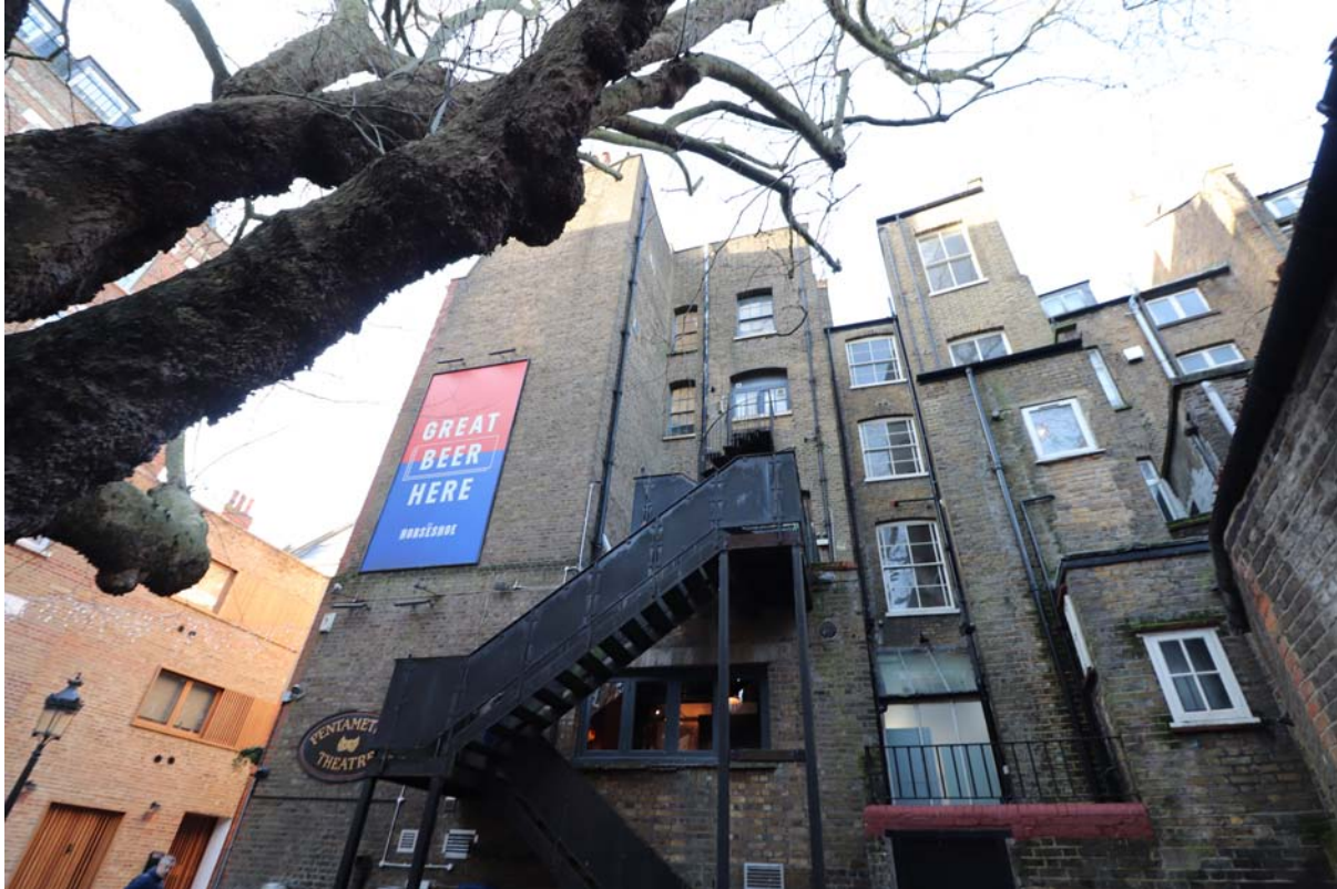
View of the existing steel fire escape from first floor to ground level.
