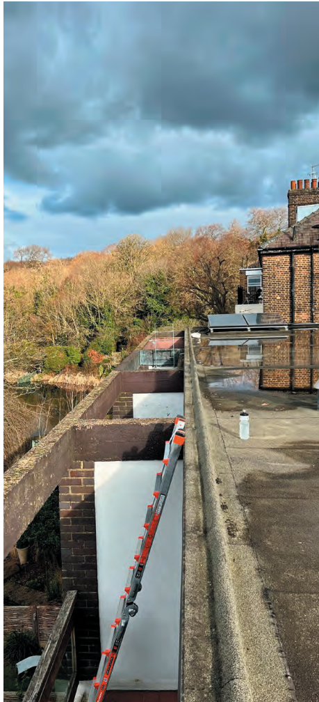
Existing unsafe roof access
