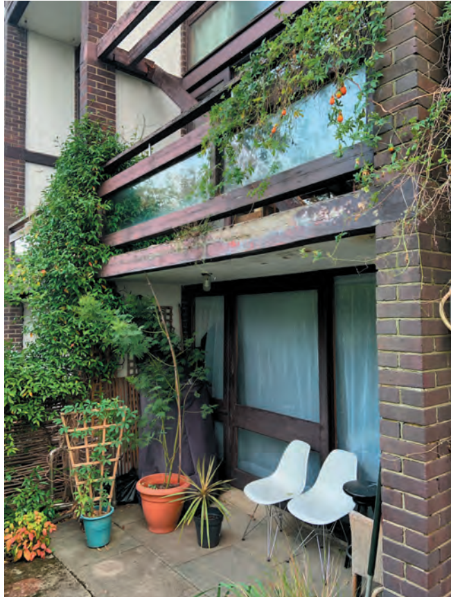
Existing rear view photos of South Hill Park showing dilapidated timber brise soleils
