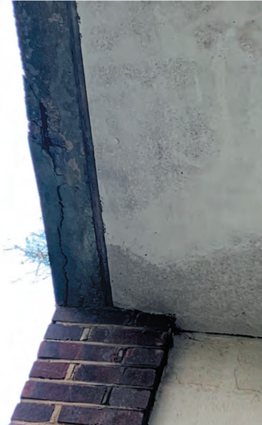
Existing rear view photos of South Hill Park showing concrete spalling and steel corrosion
