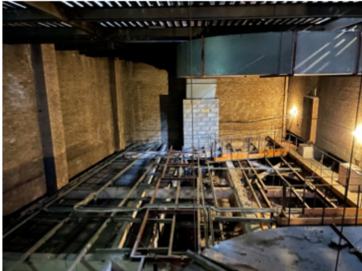
Fig 4. Fly tower used for service pipes and cables.
