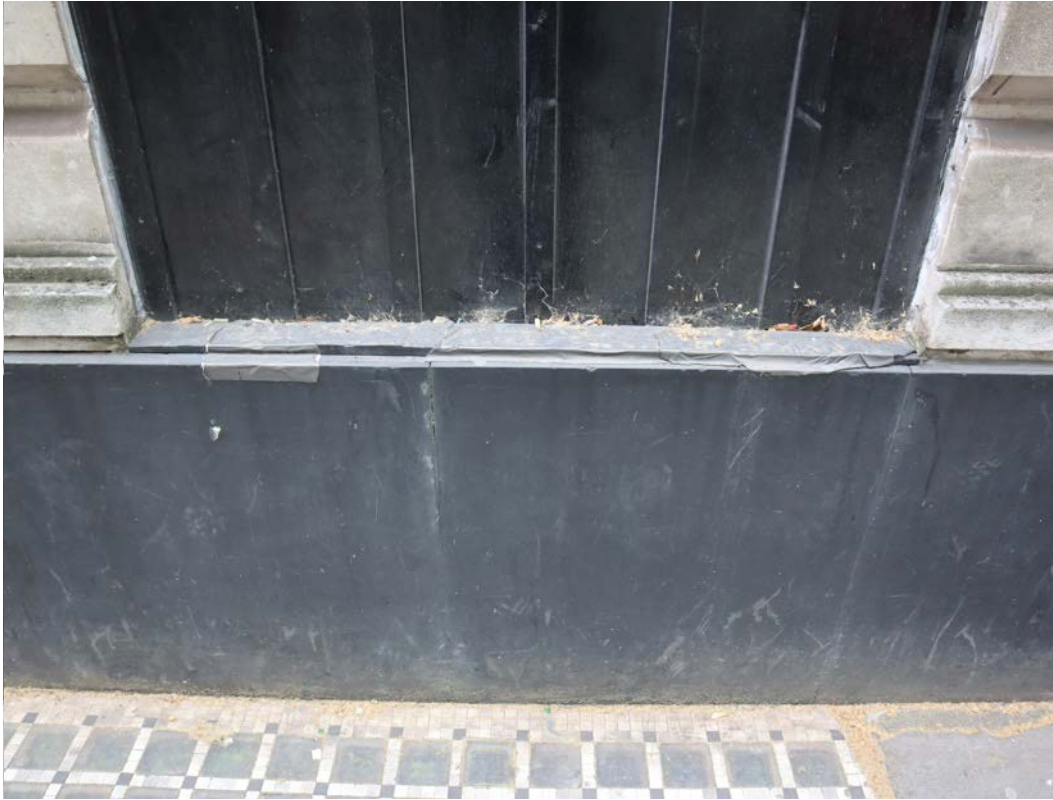
Photograph 3035. Front elevation. Damage to the slate cill has been temporarily repaired with adhesive tape
