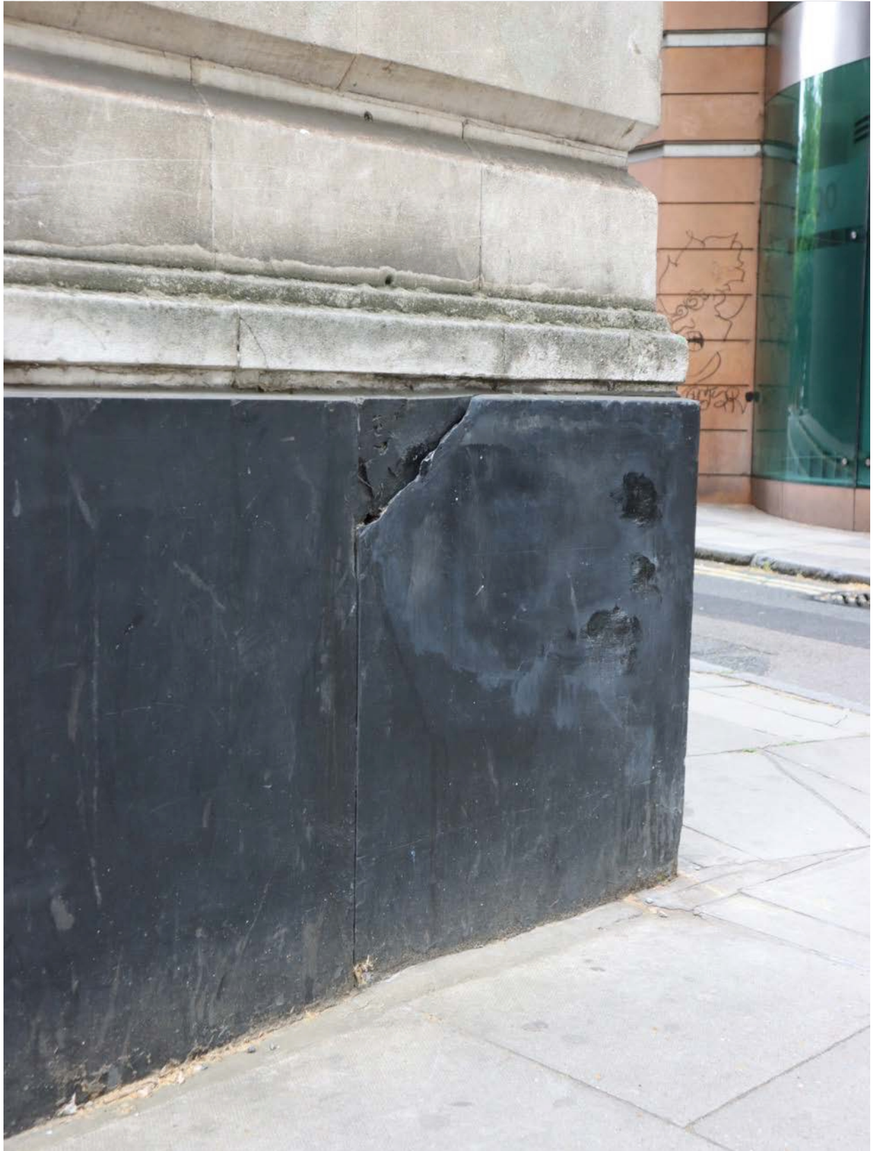
Photograph 3037. Front elevation. Damage to the slate plinth
