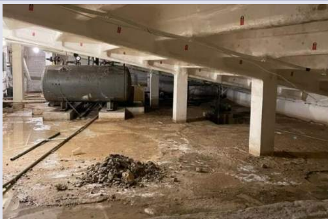
Fuel tank in basement (above and right)
