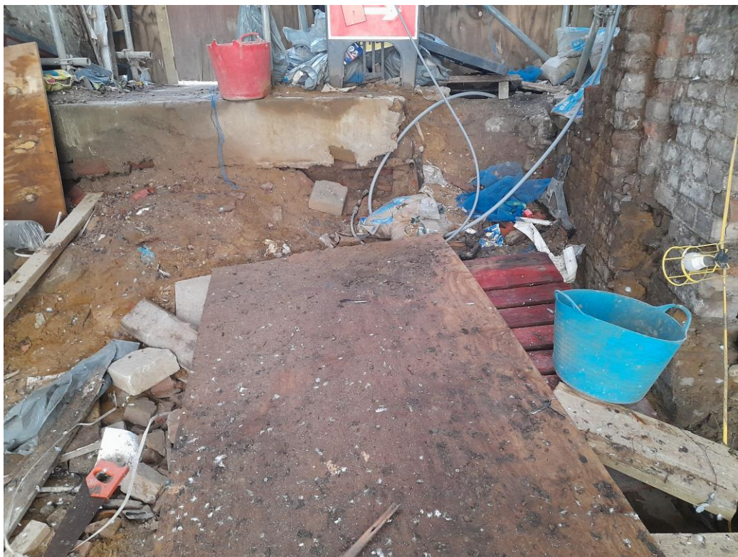
Figure 3 - Damp to debris on ground at front of property
