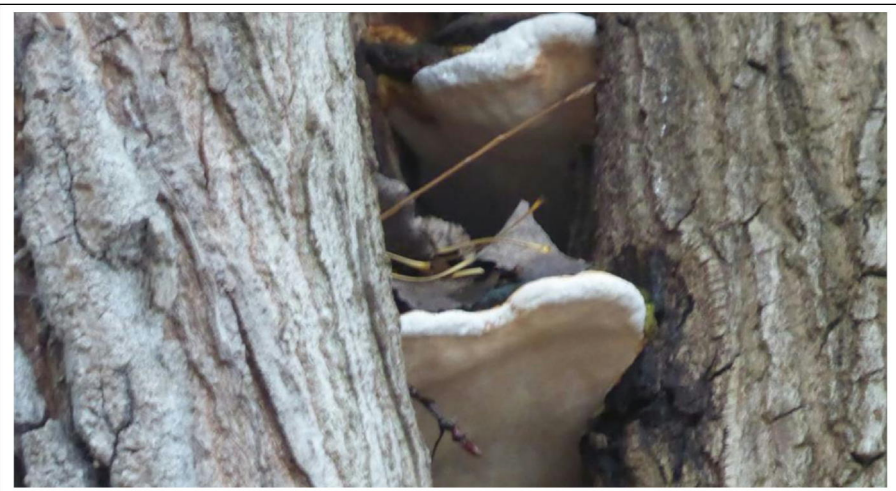
View of active fungal brackets in decay column
