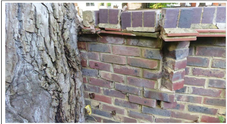
View of wall damage with main stem reaction wood encompassing wall structure
