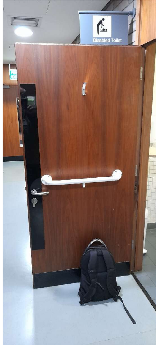
4: DDA WC door – new CPT room door to match this
