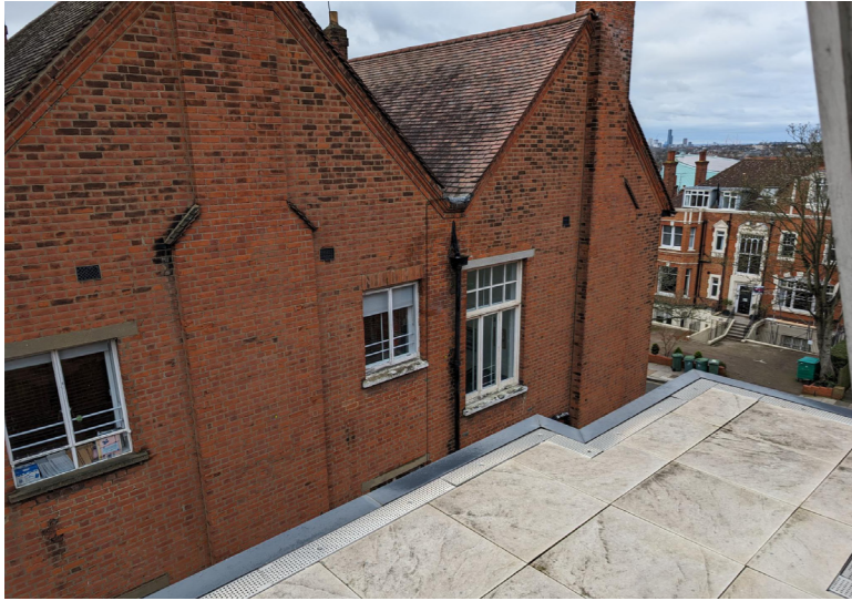
Existing flat roof outside Flat 7 with screened windows to the School opposite
