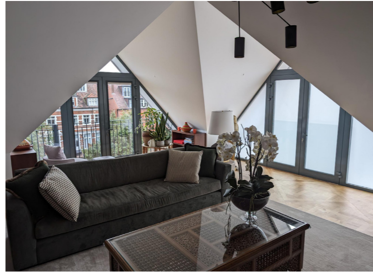
Flat 7 - existing window and doors to South elevation with obscure glass and doors out to East facing Juliette balcony
