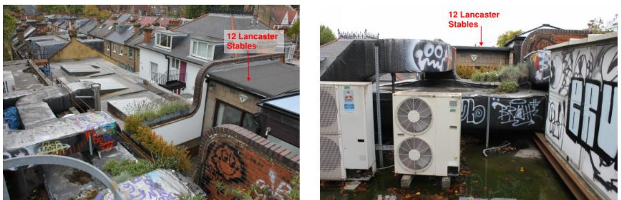
Figure 9 – photographs of 12 Lancaster Stables showing existing plant
