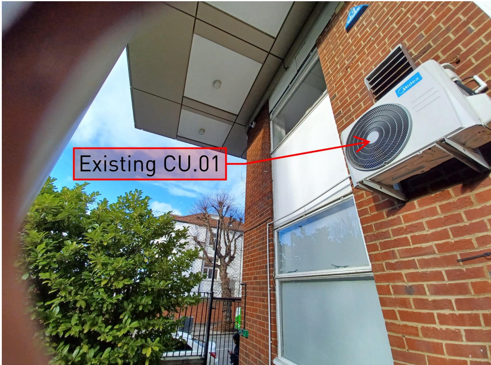
The Mulberry School, 68 Shoot Up Hill, London, NW2 Photograph of Existing Condenser Unit and Proposed Location for New Unit Project 13344
