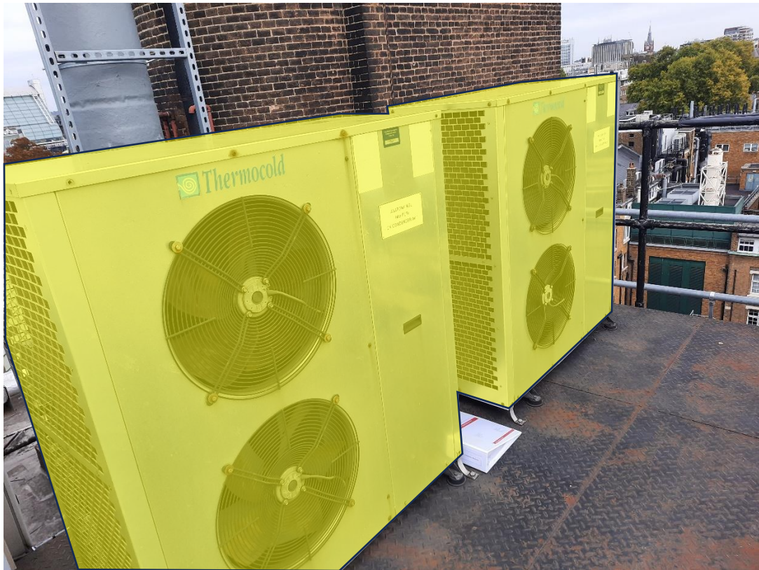
Fig 6. Existing Condenser Units to be replaced
