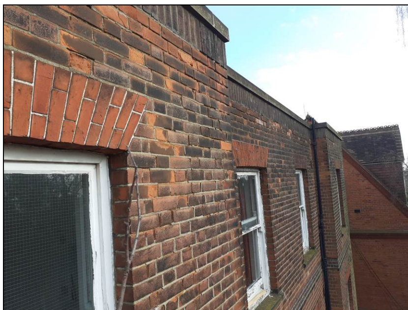
Fig 22 The exterior face of the roof parapet - as viewed from the top of the fire escape
