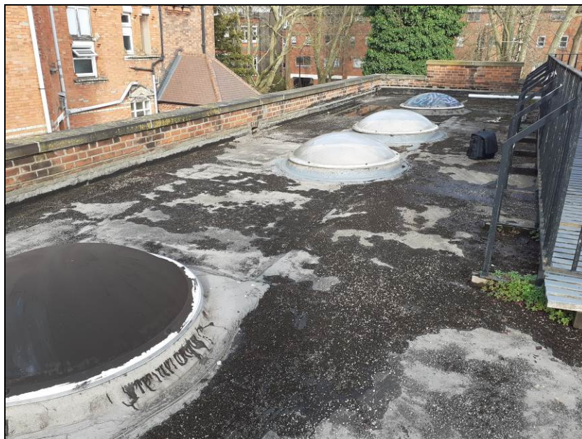
Fig 21 Roof to the two-storey northernmost part of No 39a, with light wells
