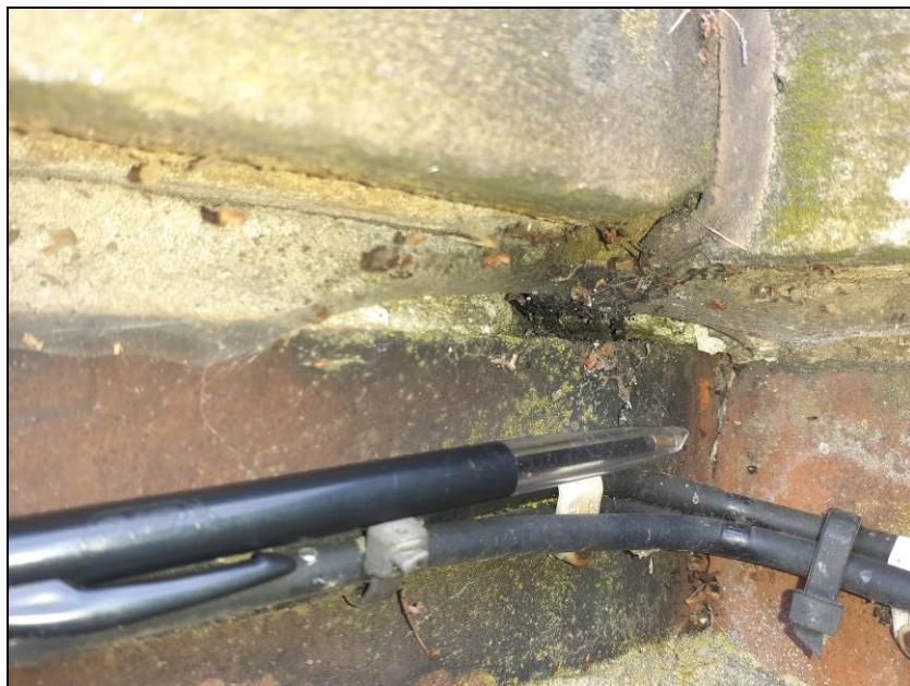
Fig 19 Mortar beneath the coping stones to the parapet mostly intact, but occasional gap is present (in this photograph, just above the tip of the pen)
