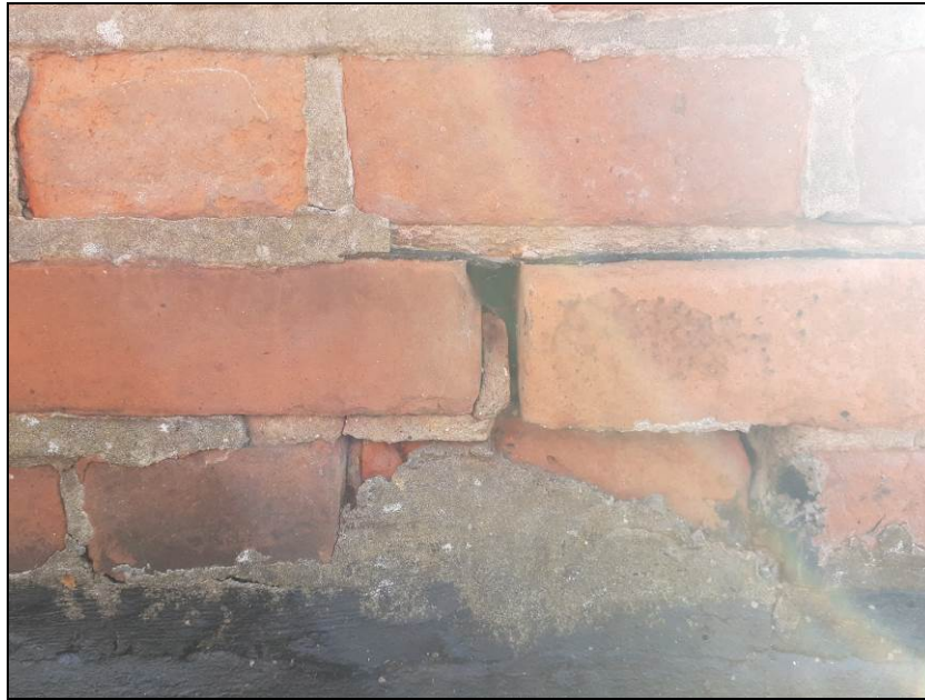
Fig 20 A rare gap in the parapet brickwork interior face
