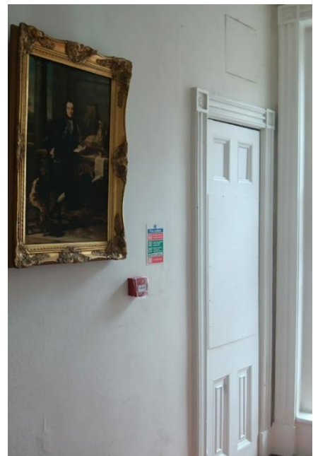
Figure 15. First floor stairwell with historic doorway in no.63 which would be removed as part of the lift installation for Option 2.
