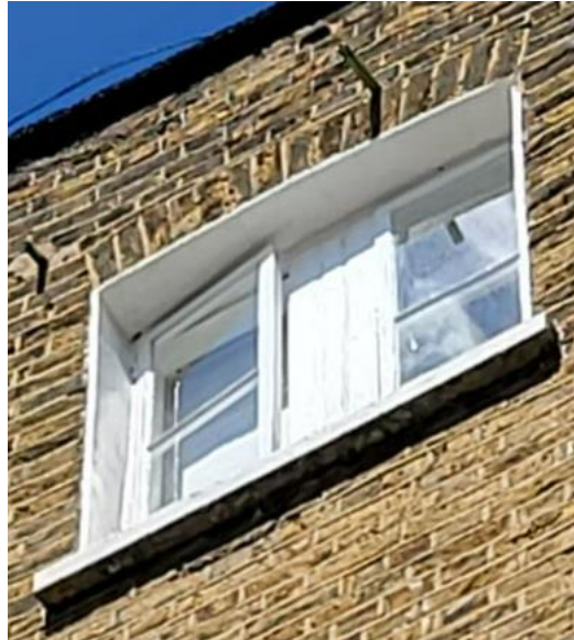
Figure 26. External view of modern casement window at third floor level proposed for removal.
