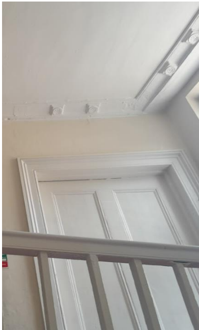
Figure 18. Second floor stairwell of no.63 showing historic cornicing that would be impacted by Option 2 .
