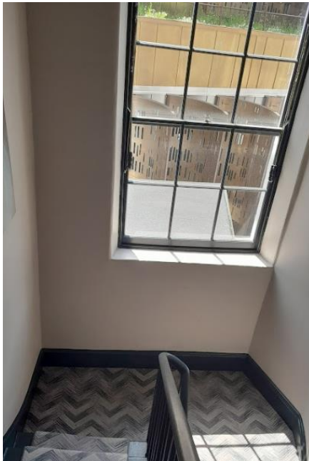
Figure 16. Second floor half landing window which would be removed to provide access to closet wing and proposed location of lift in Option 1.
