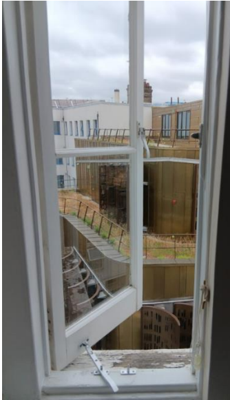
Figure 25. Internal view of modern casement window at third floor level proposed for removal
