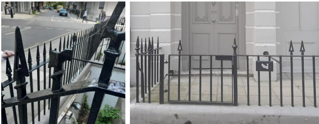
Figure 16. From left: Detail of damaged rail head ; South elevation of The Hotel on Marchmont Street with damaged railings in the foreground.
