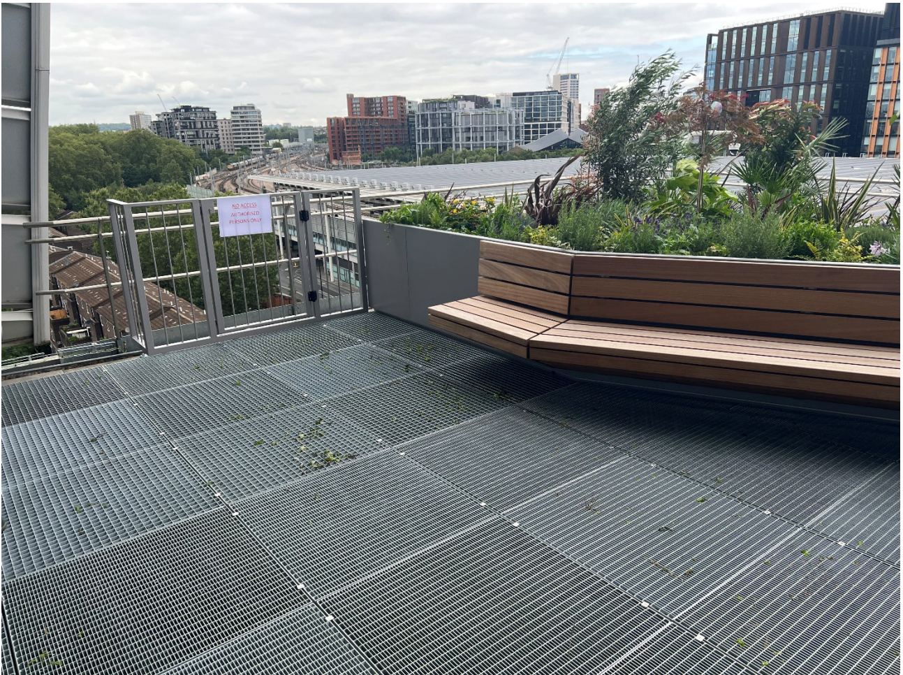
Photo – Showing maintenance gate to provide access to the edge of the Level 05 NE Terrace – This is required to remain available and necessitates the amendment to the proposed new planter at this juncture.
