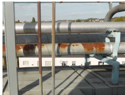
Roof mount located on Block A roof
