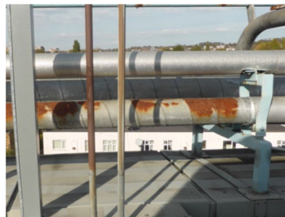
Roof mount located on Block A roof
