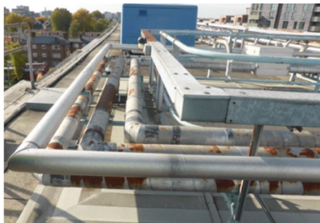
Mechanical pipes located on roof of block A
