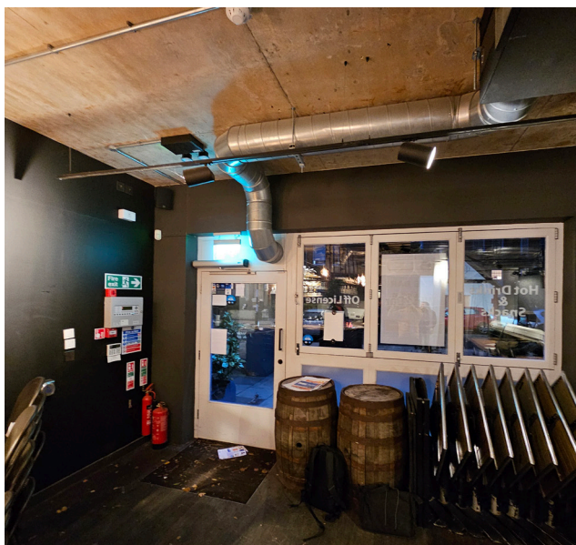
Photo 2 - Internal view towards the main entrance, with ventilation intake dropping lower than the shopfront
